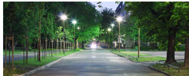
LED Streetlights © World Bank
