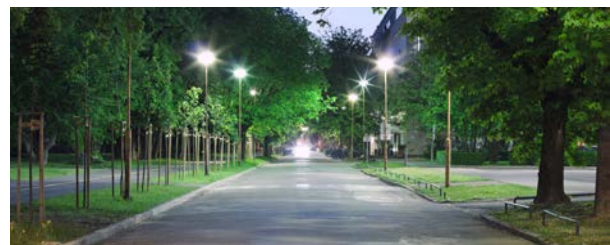
LED Streetlights © World Bank
