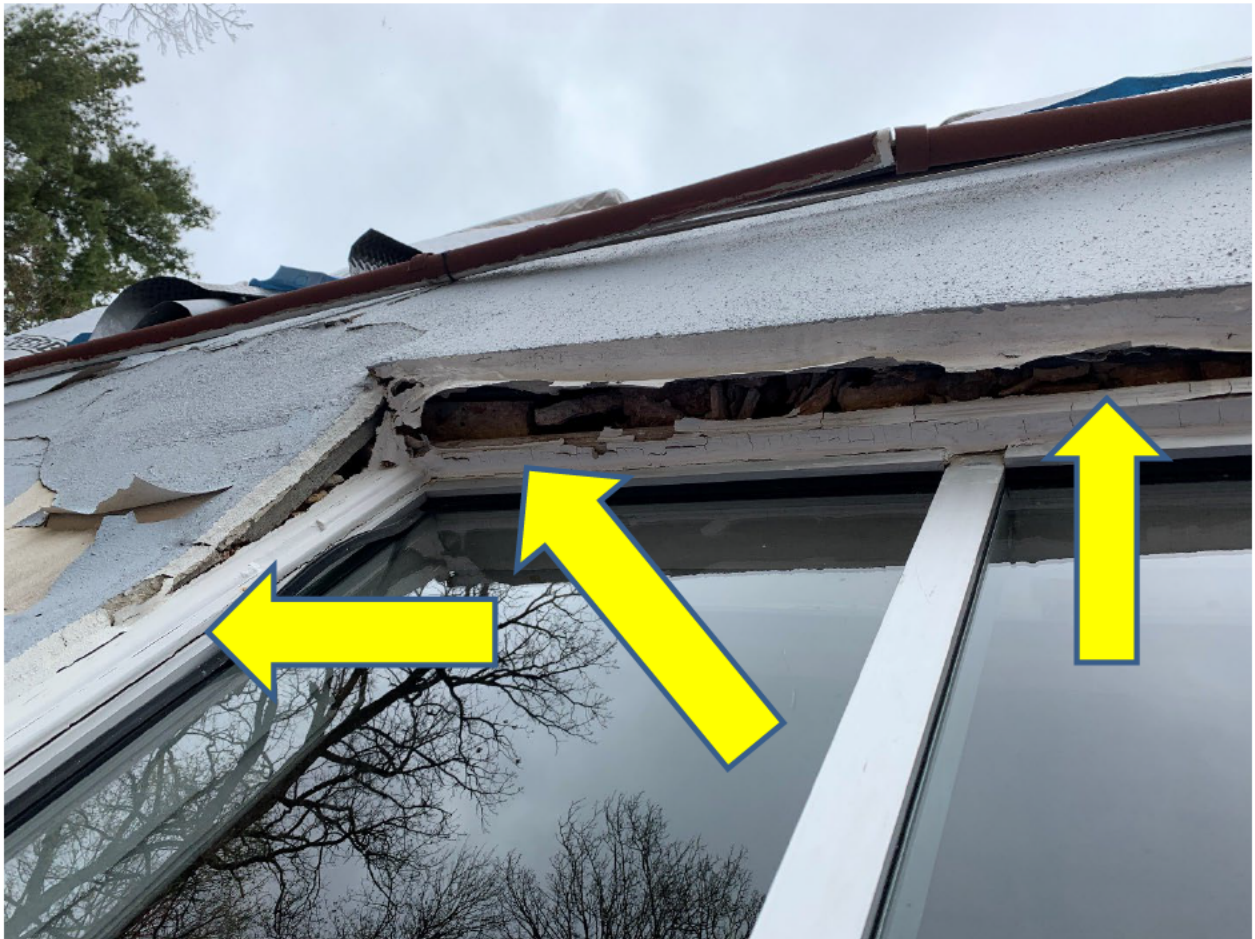
Figure 5 - close up view showing deformation of stucco at west doorway
