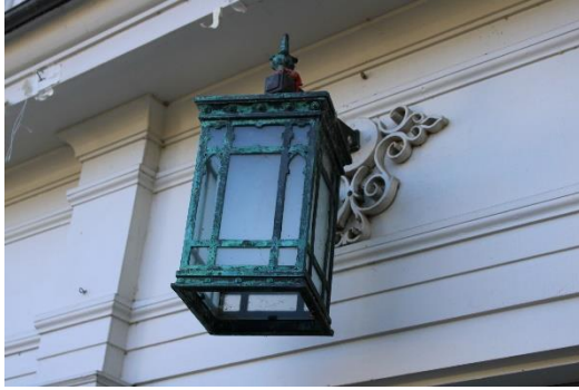
Front entrance light sconce.
