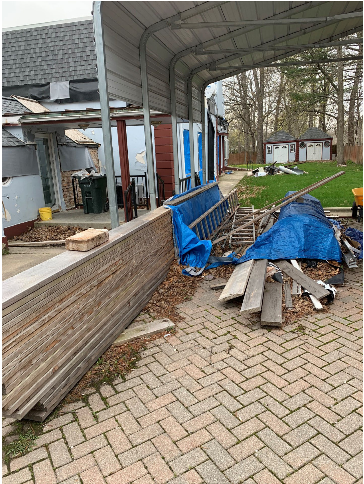
Figure 13 - site rubbish & debris
