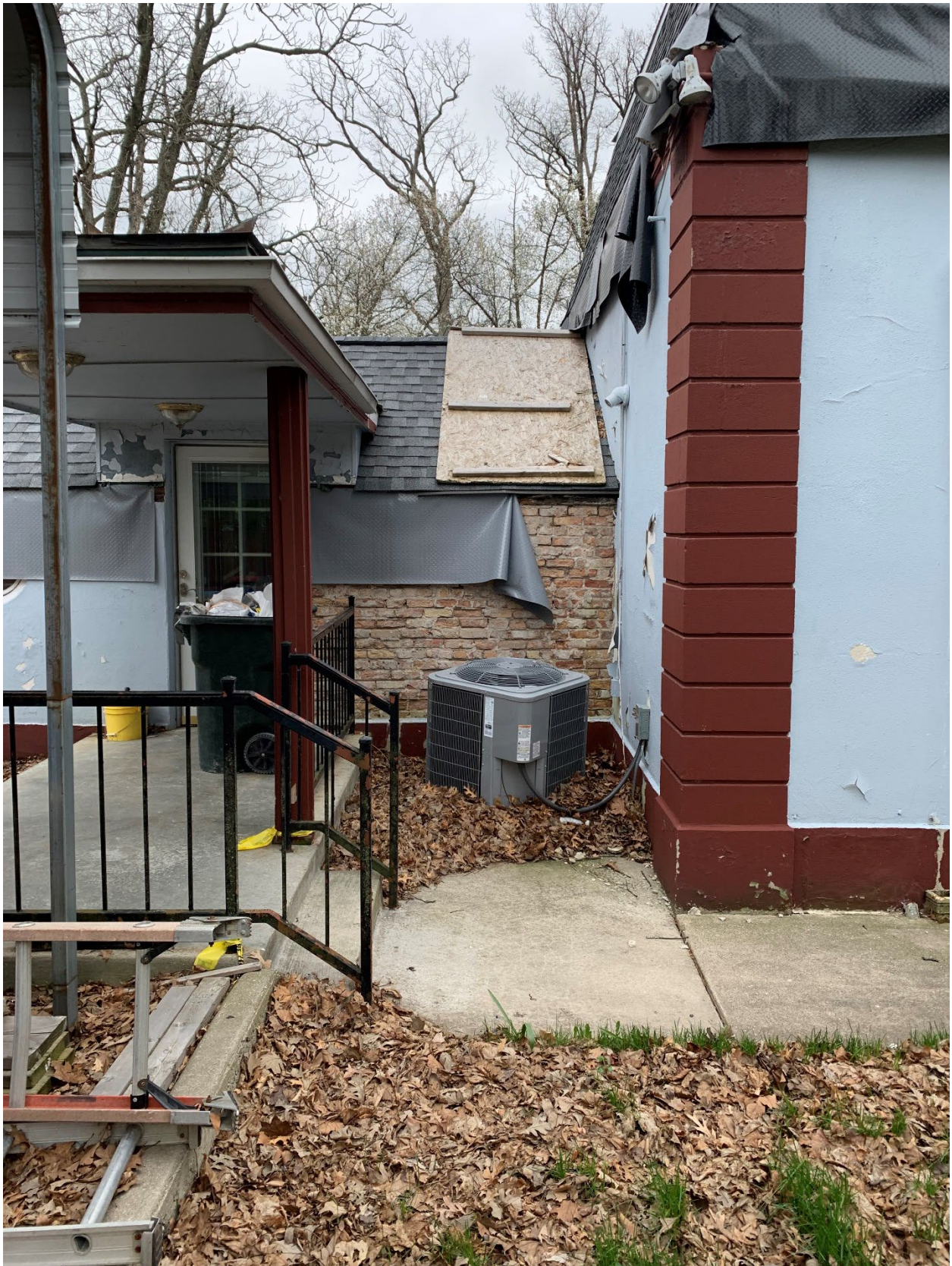
Figure 14 - inadequate temporary roof patch
