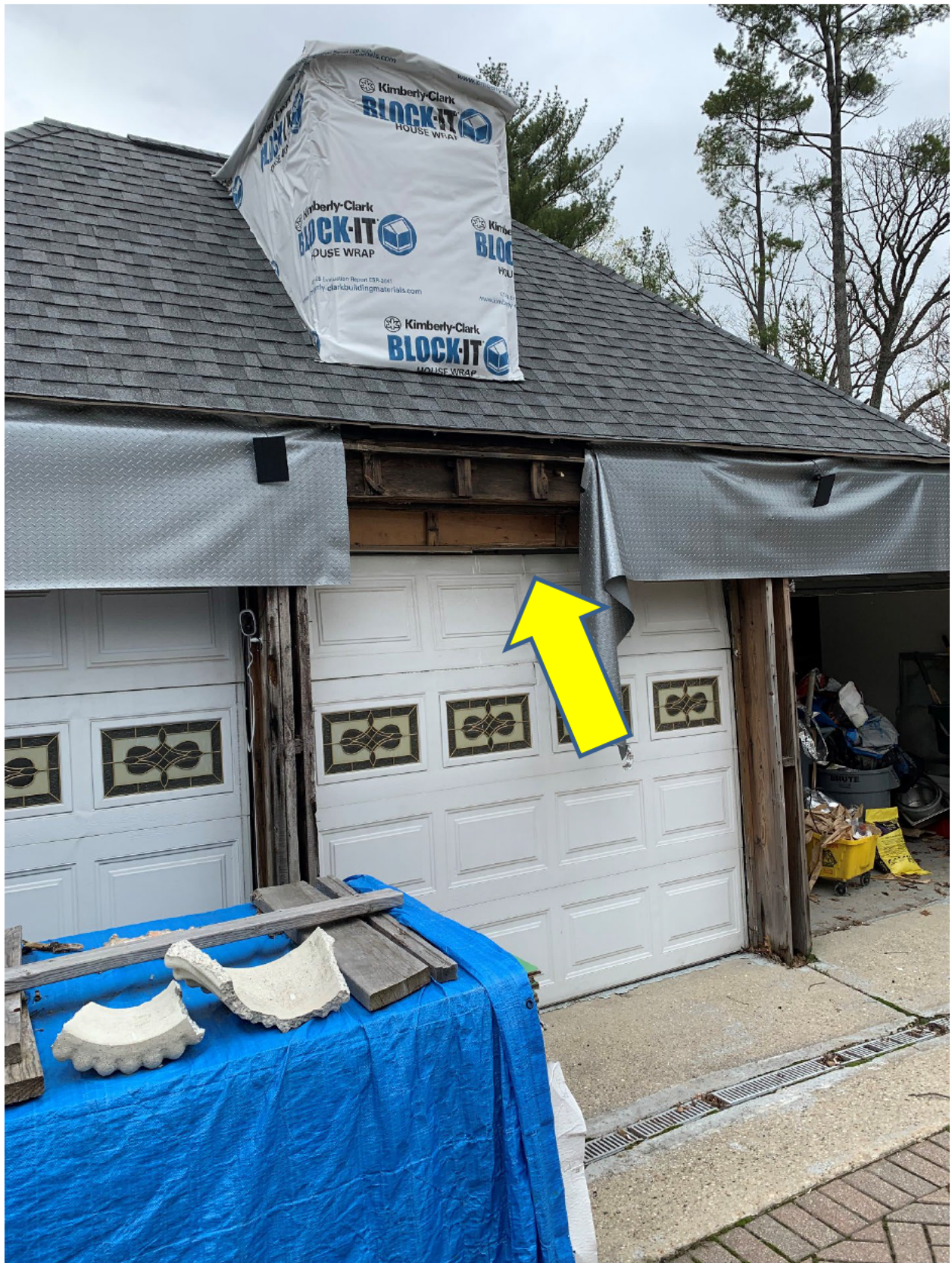
Figure 9 - unprotected garage door framing
