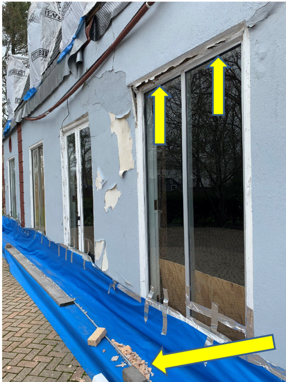
Figure 3 - damaged exterior west elevation with debris on ground
