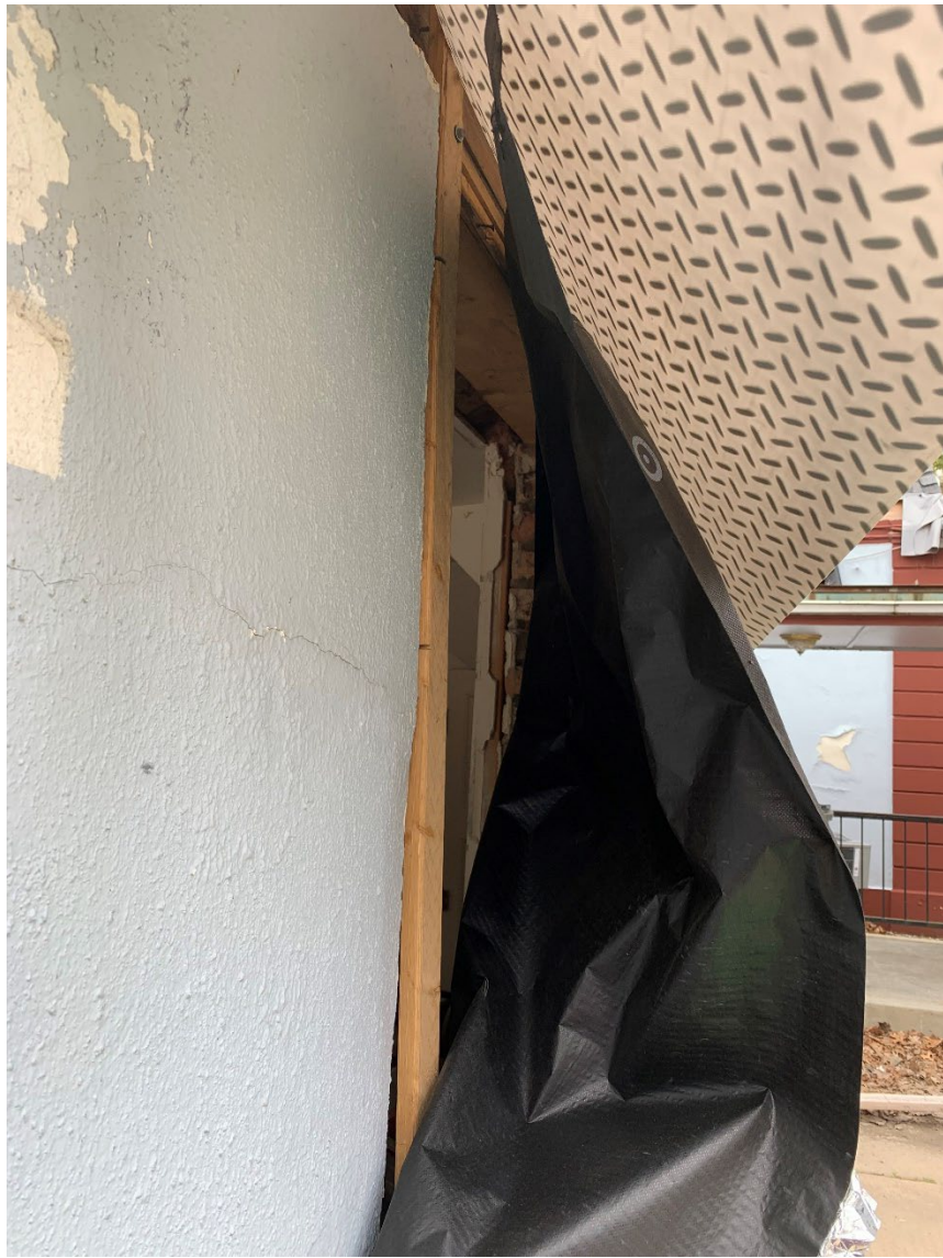
Figure 12 - unprotected garage opening
