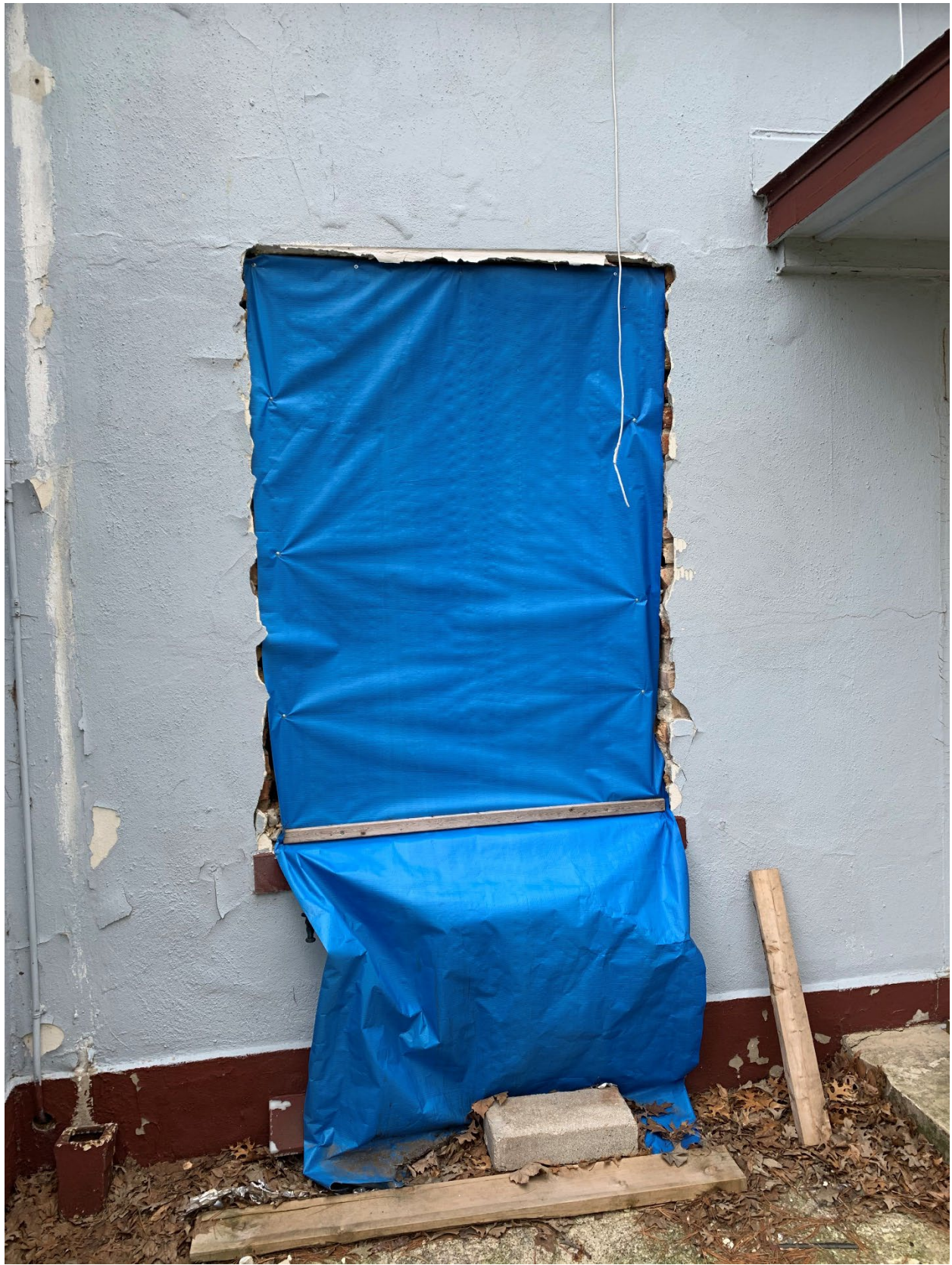
Figure 17 - inadequate protection of wall opening
