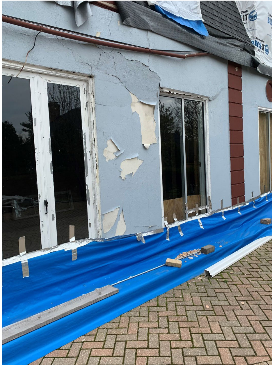
Figure 1 – area of cracked and deformed stucco (west elevation)
