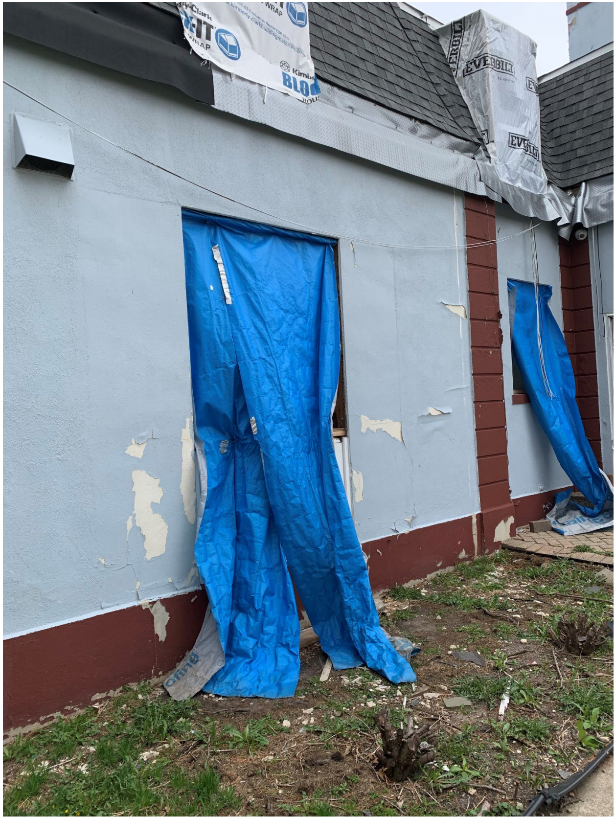
Figure 20 - inadequate protection of window openings
