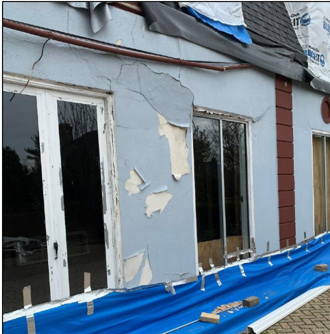
Cracked and deformed stucco on rear façade. (Village of Winnetka)
