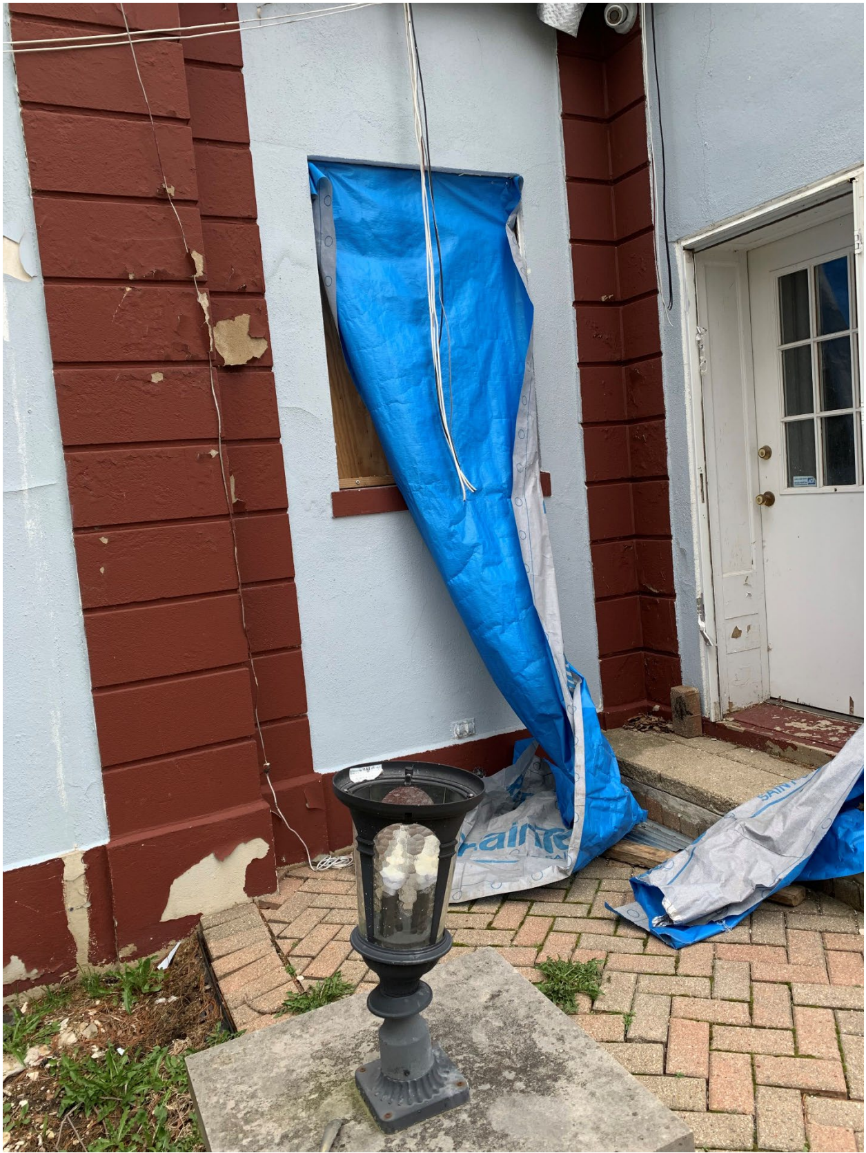
Figure 21 – poorly protected opening
