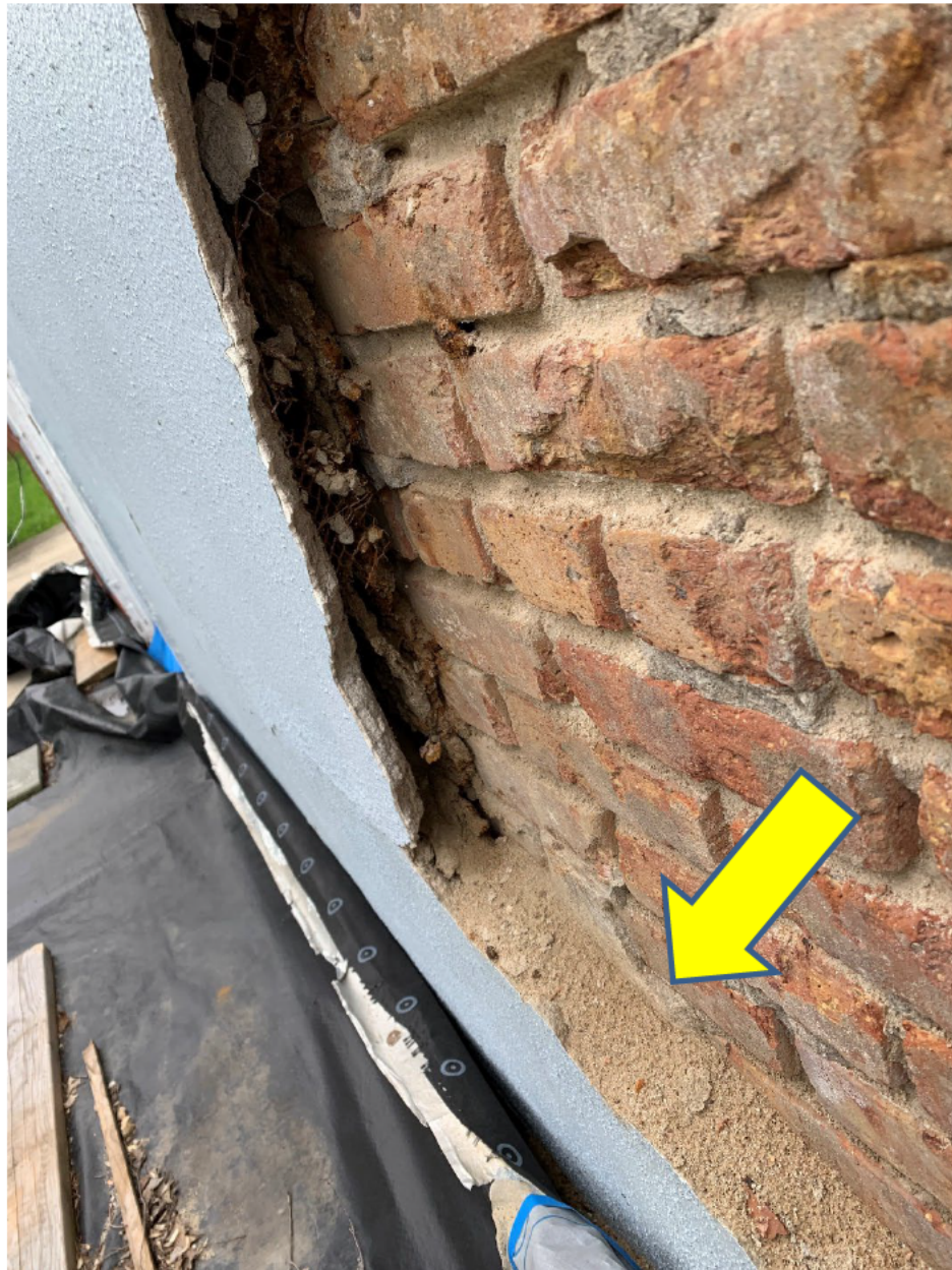
Figure 8 – erosion of mortar (sand) collected at stucco failure
