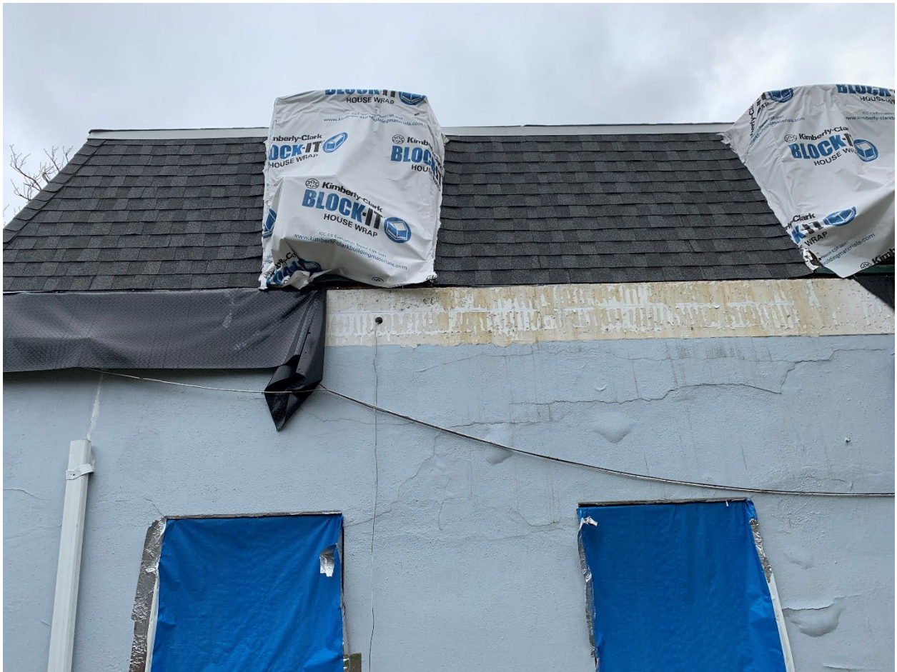
Figure 15 - missing/damaged temporary protection from water entry
