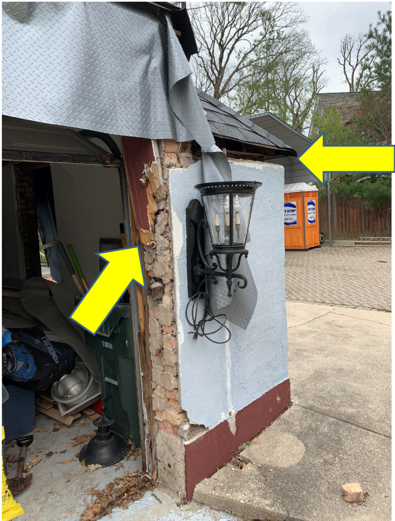
Figure 10 - Damaged garage door wall, gap at top of wall
