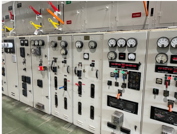
Photo: North – South 4kV Bus
