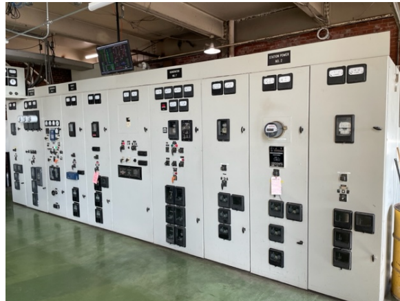
Photo: East 4kV Bus
