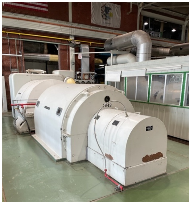
Photo: Steam Turbine #6
