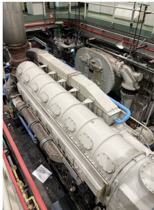
Photo: Diesel Generator #8
