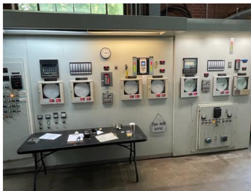
Photo: Boiler Controls
