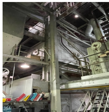
Photo: Lower Section of Boiler
