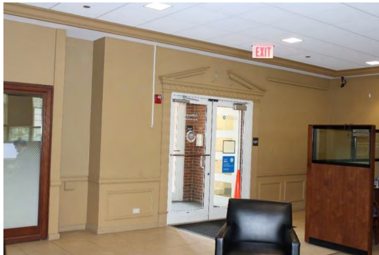
South entrance showing broken pediment and chair railings.
