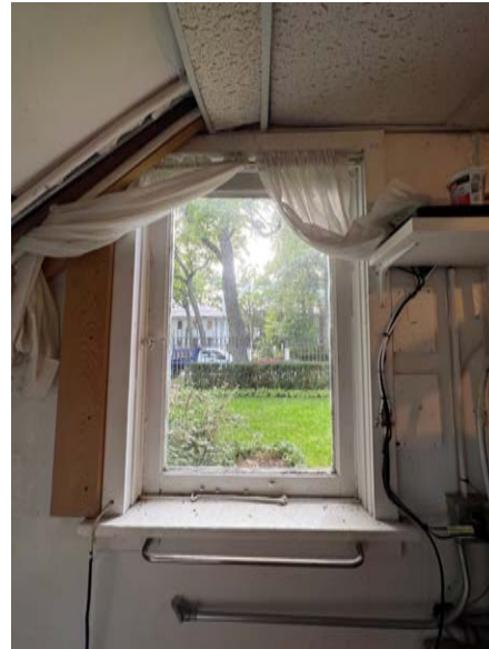
Window in mechanicals room
