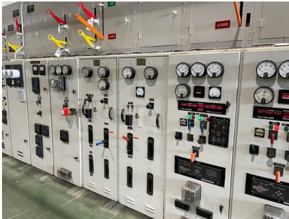
Photo: North – South 4kV Bus
