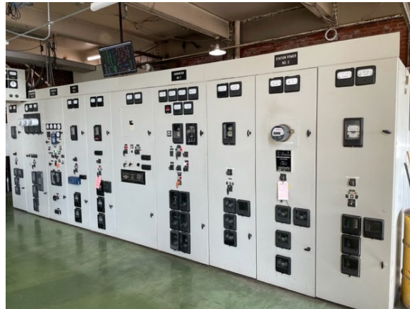
Photo: East 4kV Bus
