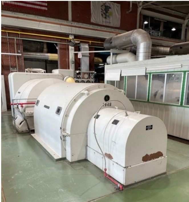
Photo: Steam Turbine #6
