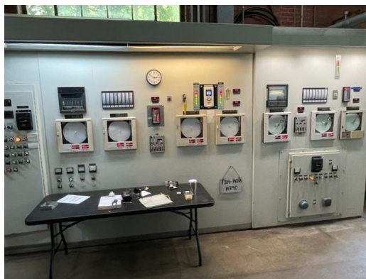
Photo: Boiler Controls
