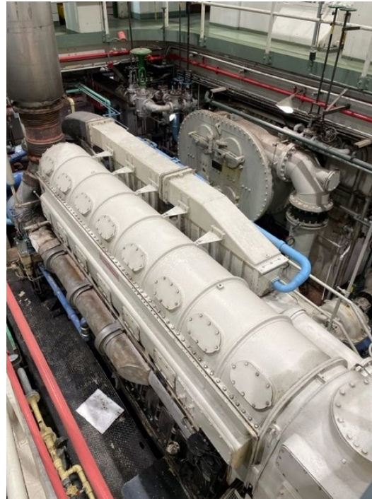
Photo: Diesel Generator #8
