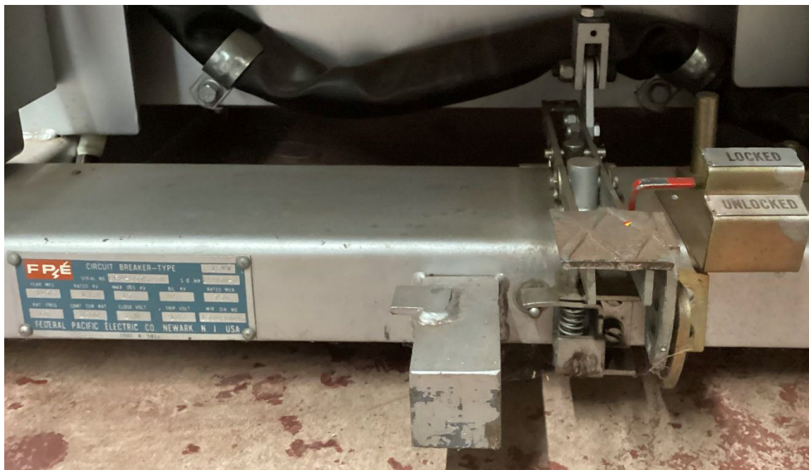
5.6 Federal Pacific Breaker Interlocking device
