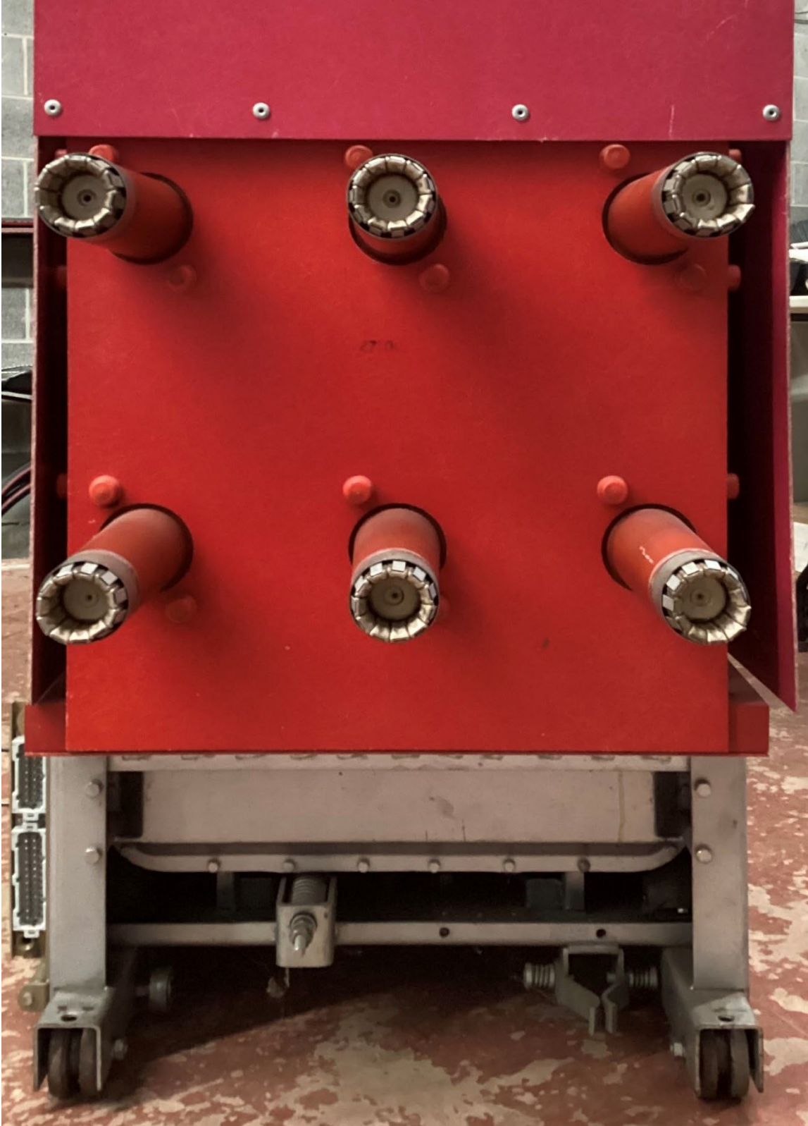
5.4 Federal Pacific Breaker rear view
