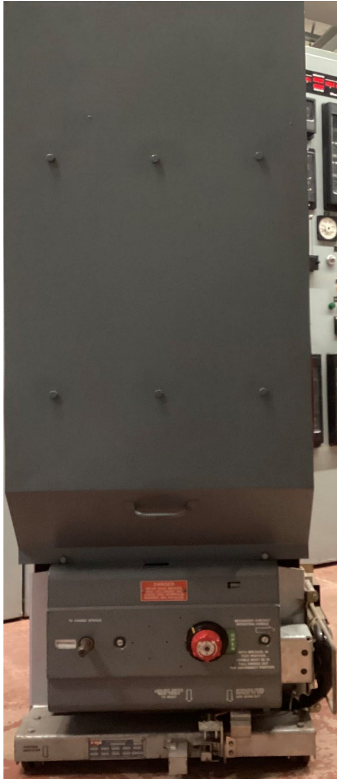
5.1 Federal Pacific Breaker
