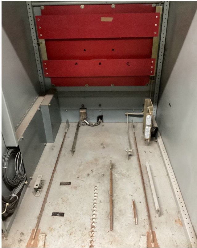
5.10 Federal Pacific Breaker cubicle
