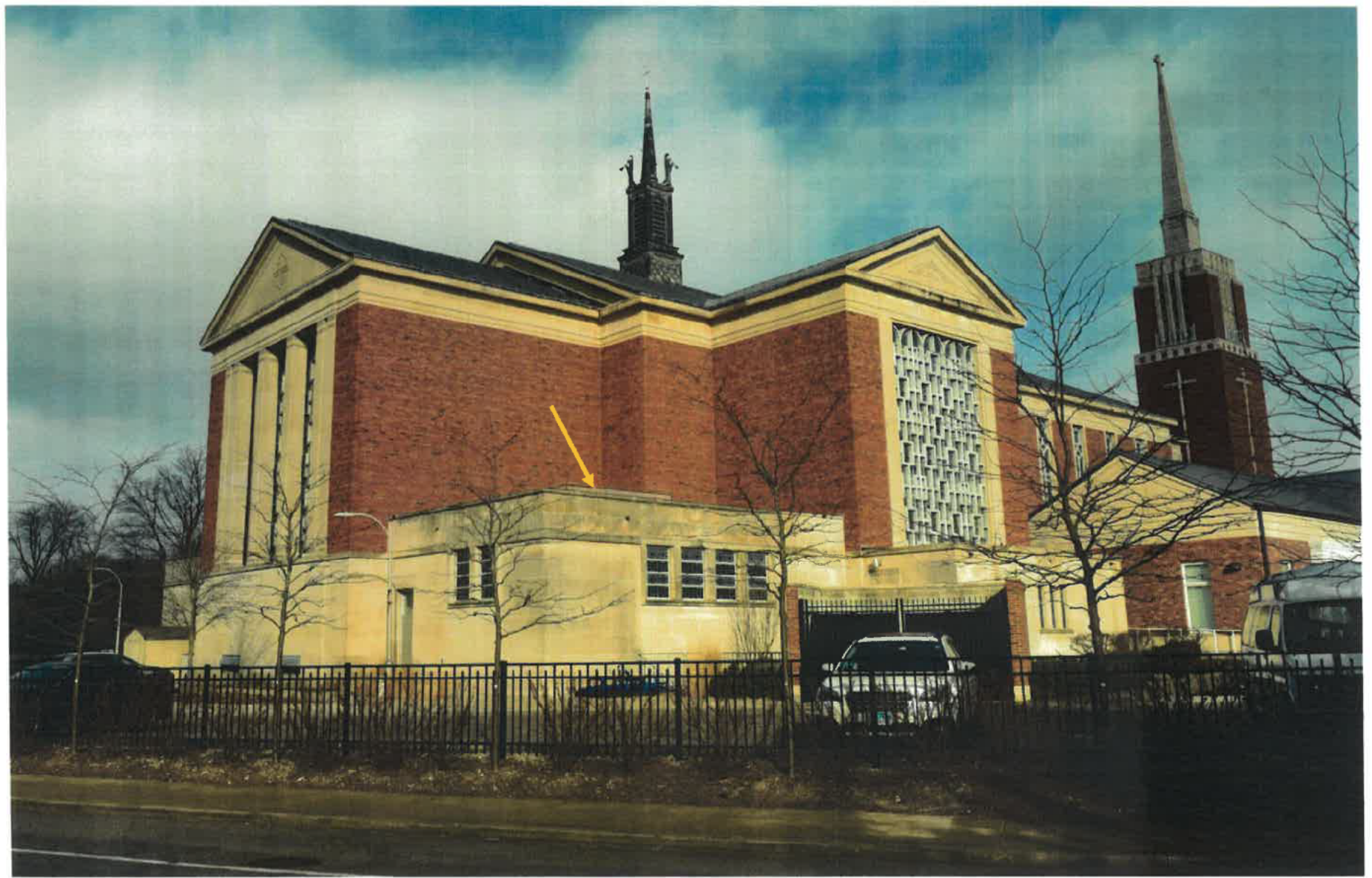
NEW CONDENSER UNIT(S) AS SEEN FROM SOUTHEAST (FROM CENTERLINE OF HILL ROAD)
