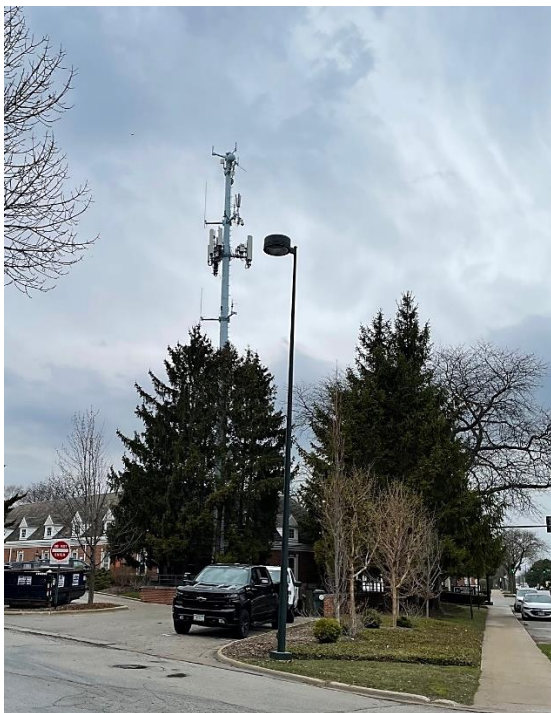
Monopole from Ash Street & Green Bay Road
