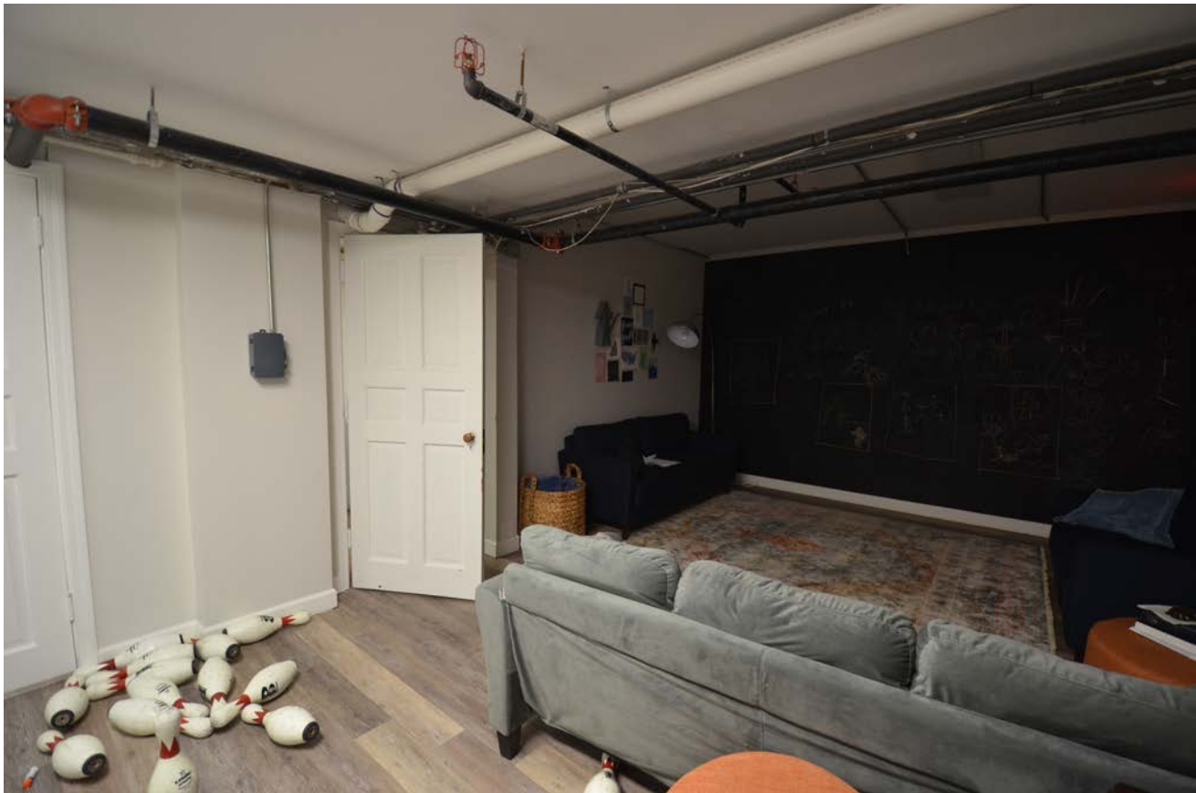
LIMITED HEADROOM IN EXISTING BASEMENT
