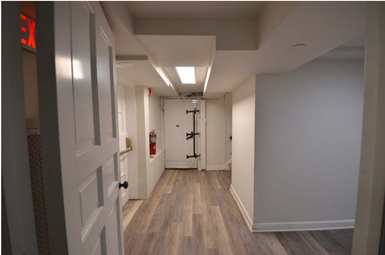
LIMITED HEADROOM IN EXISTING BASEMENT
