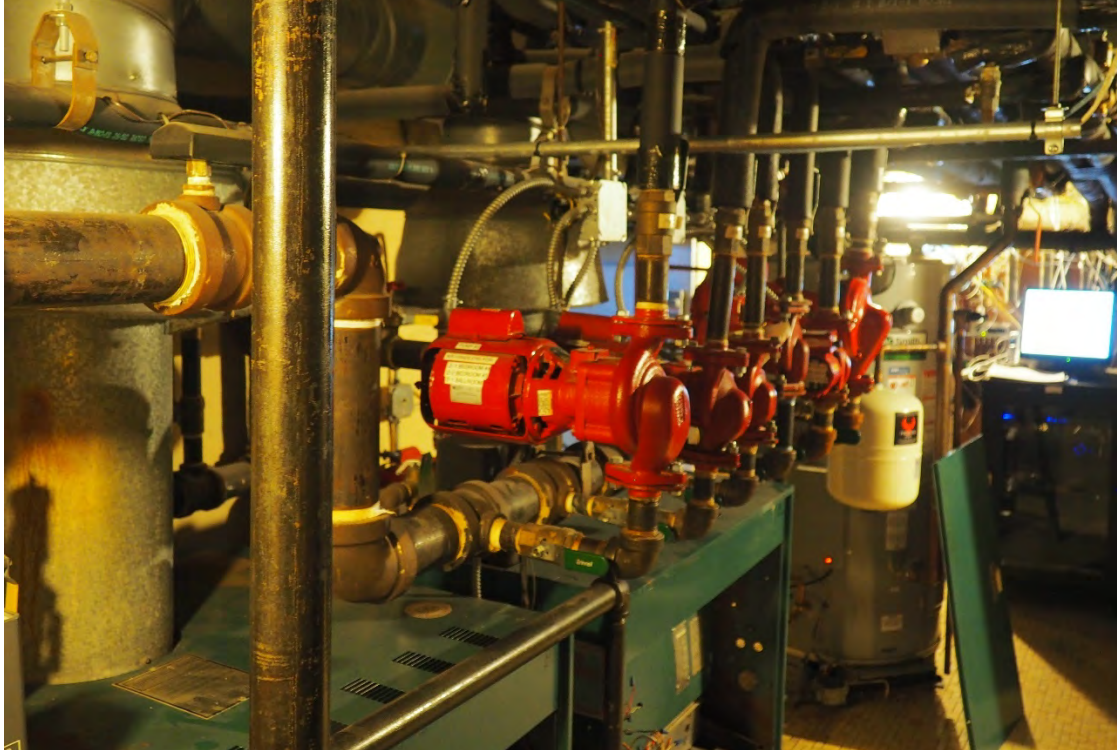
Photograph 20: View of the basement electrical room looking south, 2024.
