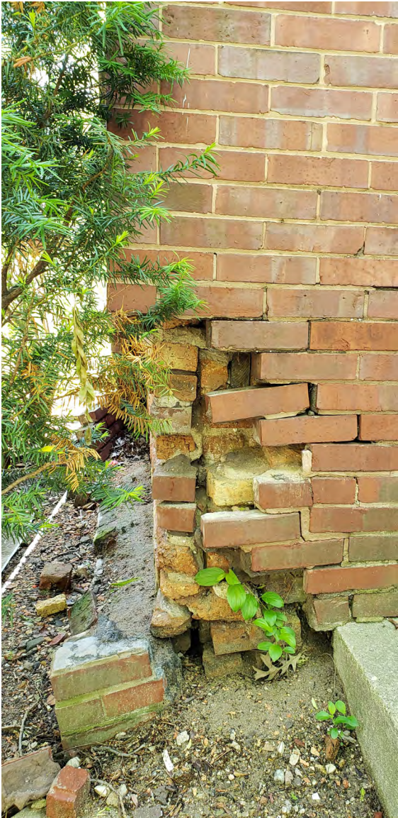
SUBSTANTIAL MASONRY DAMAGE NOTED AT MULTIPLE CORNERS. LIKELY DUE TO SETTLEMENT OF FOUNDATION.
