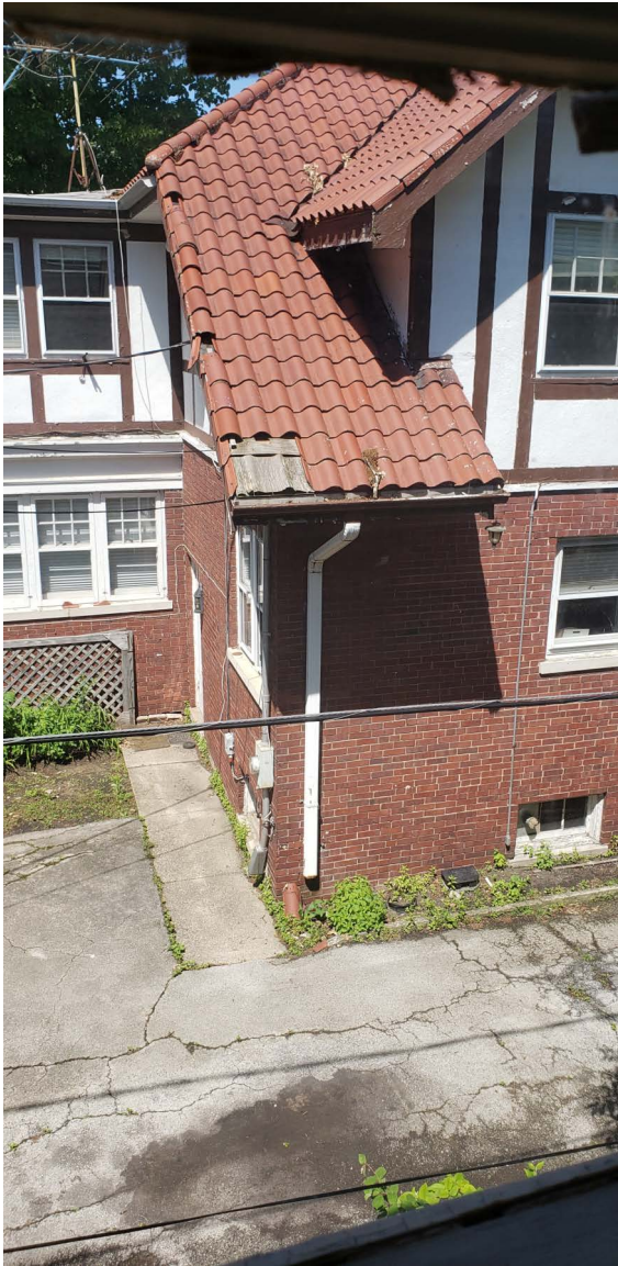
MISSING AND DAMAGED CLAY ROOF TILES
