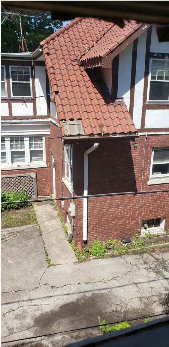
MISSING AND DAMAGED CLAY ROOF TILES
