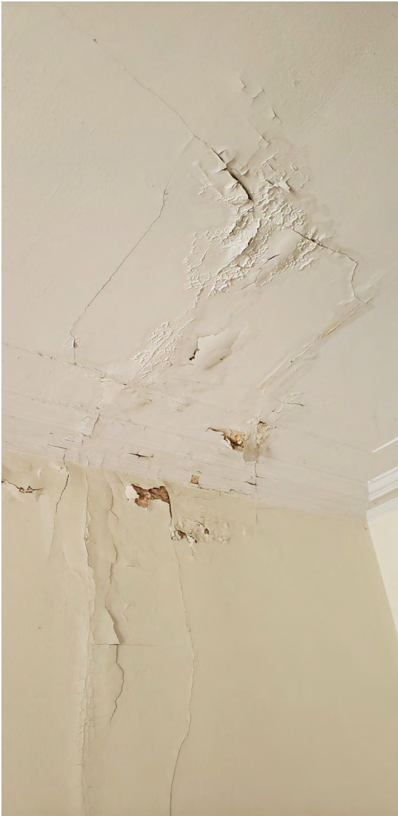
WATER DAMAGE THROUGHOUT SECOND FLOOR CEILING DUE TO DISREPAIR OF ROOF
