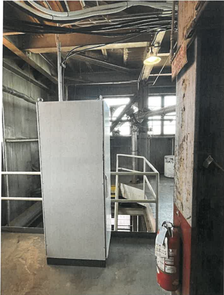
Red Center Equipment Enclosure
