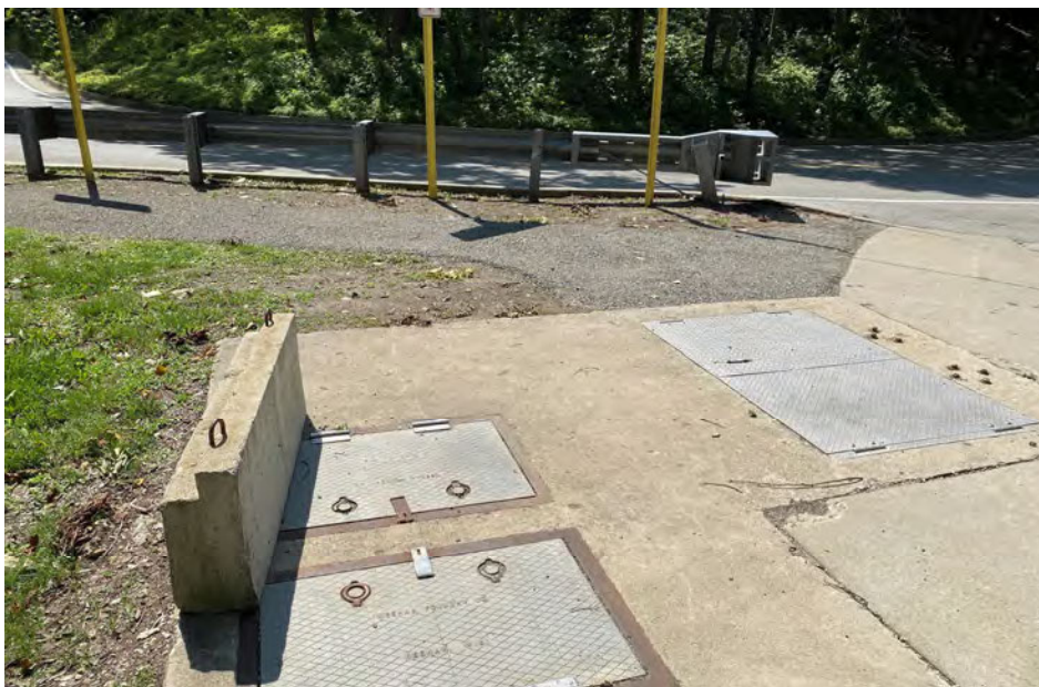
The existing Ravines Lift Station submersible pumping station along Sheridan Road.
