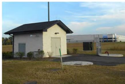
Bluff Road sanitary pumping station.
