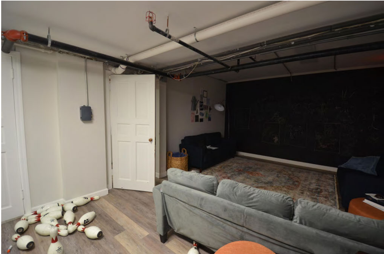
LIMITED HEADROOM IN EXISTING BASEMENT
