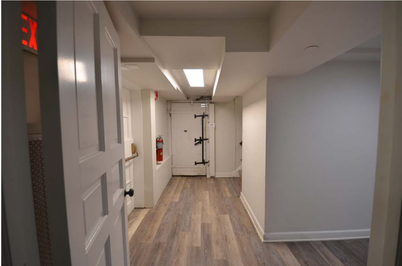
LIMITED HEADROOM IN EXISTING BASEMENT
