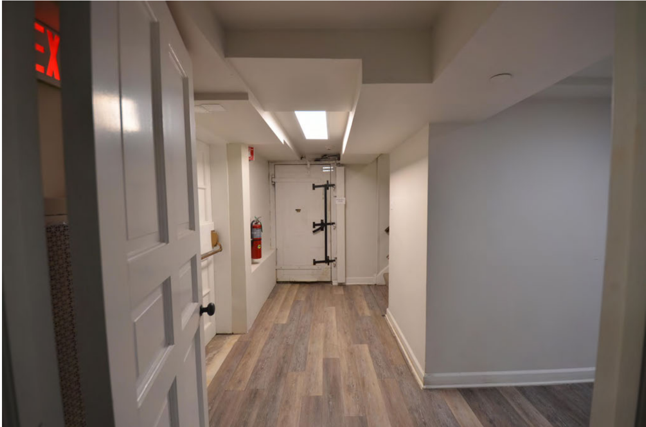
LIMITED HEADROOM IN EXISTING BASEMENT
