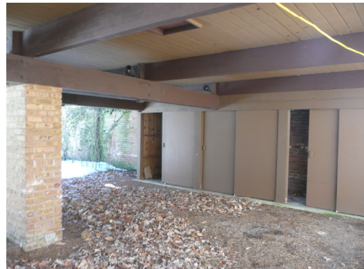
Carport bicycle storage
