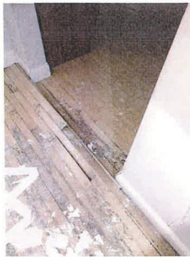
Photo 1h: Mold growth and water damage visible on the hardwood floors.
