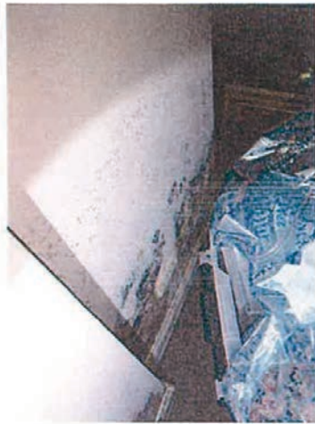
Photo 1i: Mold growth visible in the rear sitting area of the home.
