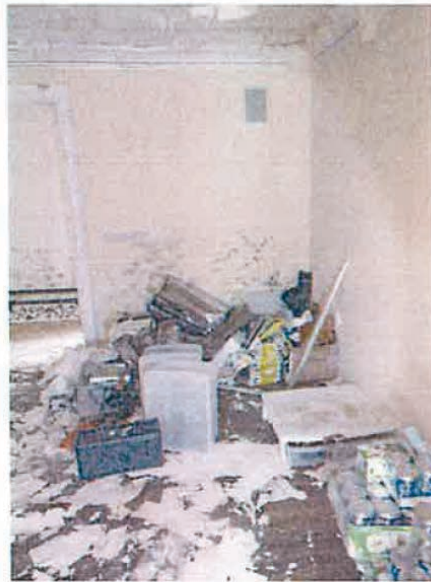
Photo 1b: Mold growth visible on the drywall in the living room.
