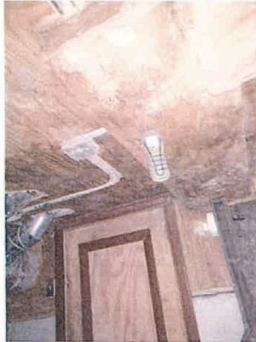
Photo 2g: Moisture on the ceiling in the basement.
