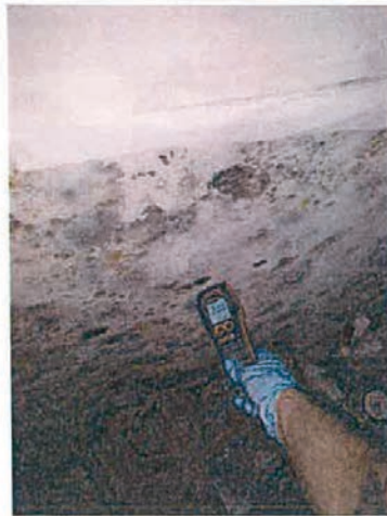
Photo 2a: Moisture on the drywall in the rear sitting room.
