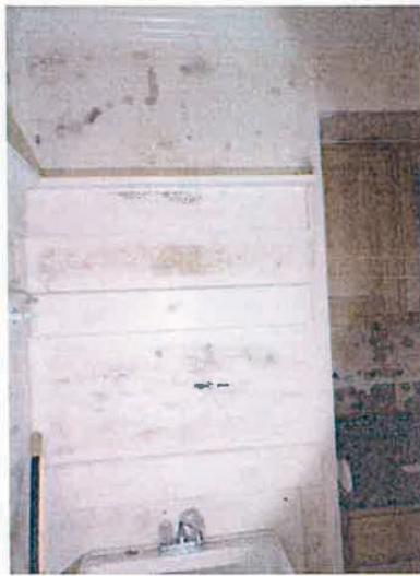
Photo 1f: Mold growth visible throughout the laundry room.
