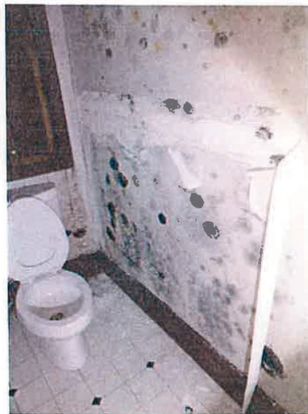
Photo 1c: Mold growth visible in the hall bathroom on the 1st floor.
