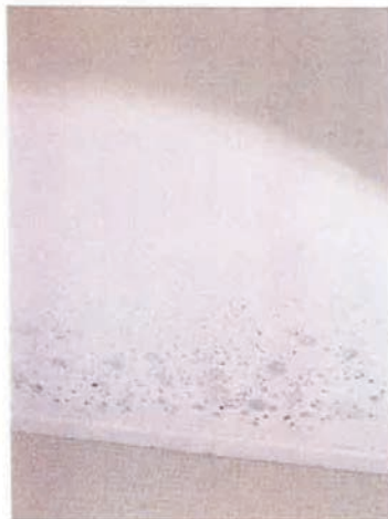
Photo 1k: Mold growth visible on the drywall in closets on the 2nd floor.
