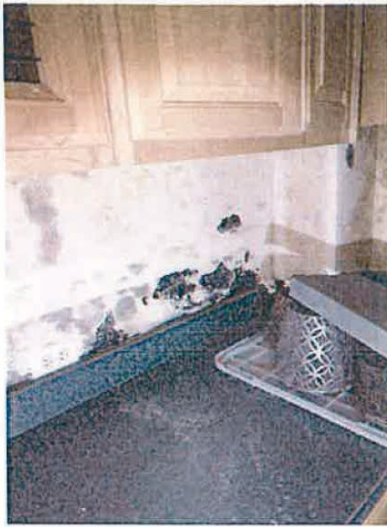
Photo 1e: Mold growth visible throughout the laundry room.
