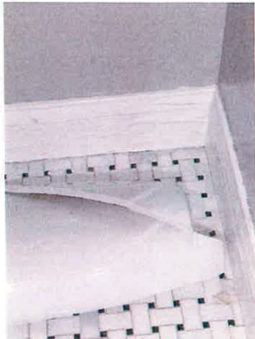
Photo 2i: Water damage visible on baseboards and drywall in a bathroom on the 2nd floor.
