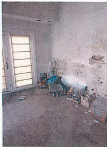
Photo 1j: Mold growth visible in the rear sitting area of the home.
