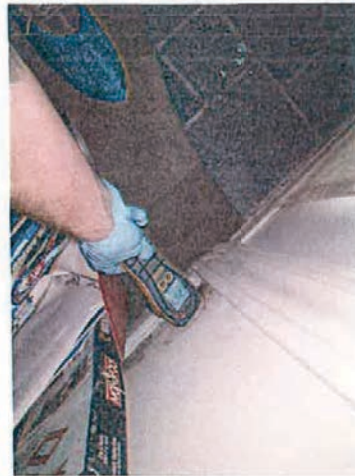
Photo 2b: Moisture on the drywall in the rear sitting room.
