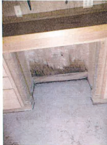
Photo 2h: Moisture underneath a workbench in the basement.
