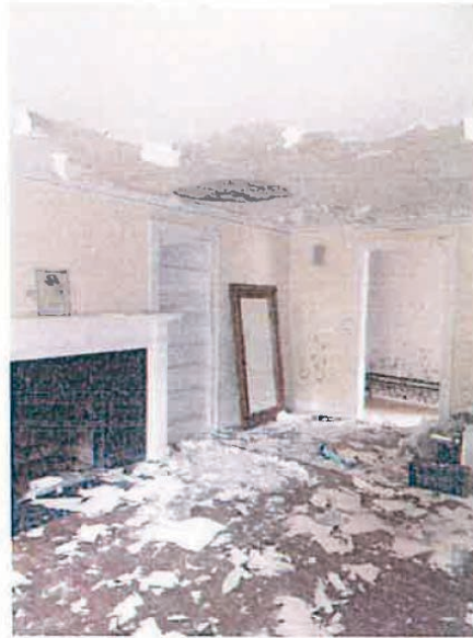
Photo 1a: Mold growth visible on the drywall in the living room.
