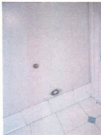
Photo 1l: Mold growth visible on the drywall in a bathroom on the 2nd floor.
