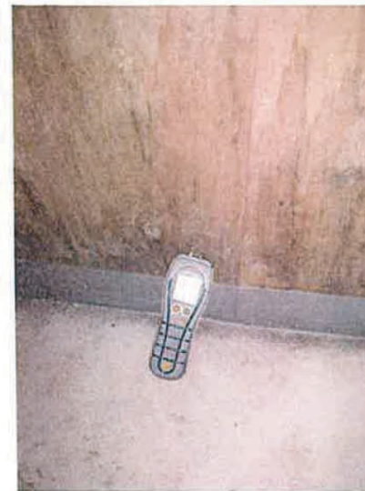
Photo 2f: Moisture on plywood walls in basement.
