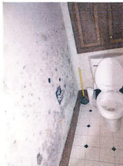
Photo 1d: Mold growth visible in the hall bathroom on the 1st floor.
