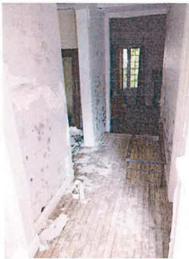
Photo 1g: Mold growth visible in the hallway on the floor and drywall.
