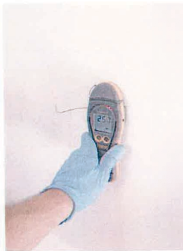
Photo 3b: A moisture meter indicating that the ceiling is damp.
