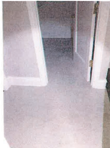
Photo 2j: The floor underneath the carpet was buckled on the 2nd floor outside of the bathroom.
