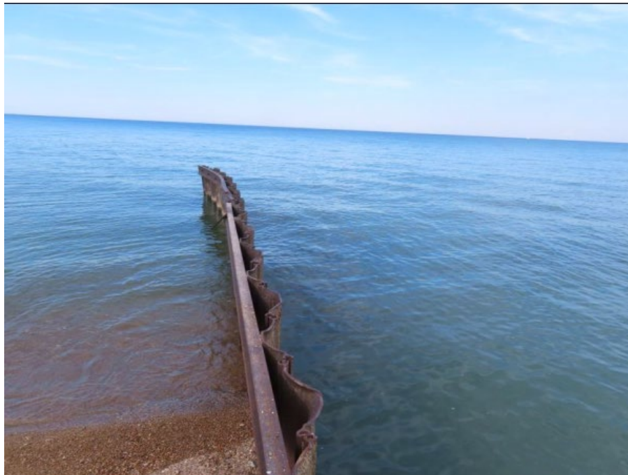
Existing Central Groin Structure Failure Progression
