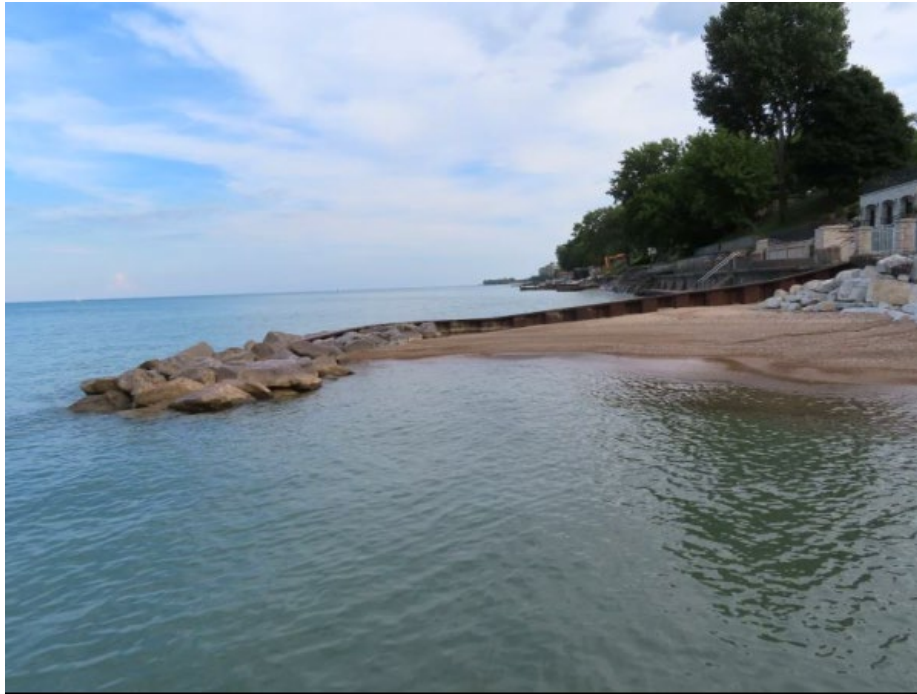
Existing South Groin, Beach Erosion and Damaged Breakwater
