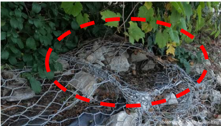
Damaged gabion basket
