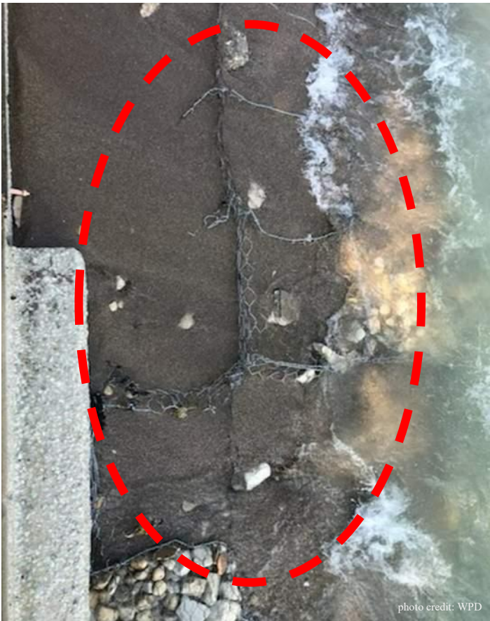
Damaged gabion baskets
