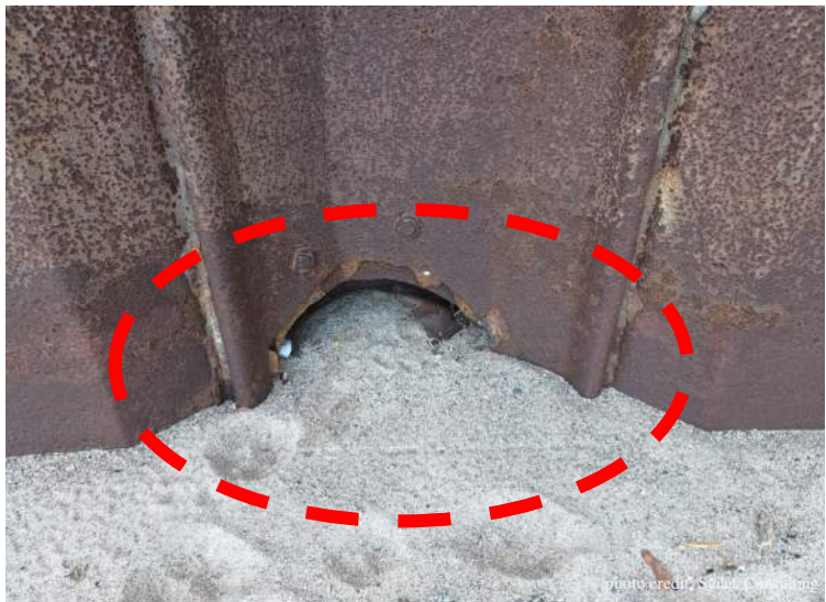
Damaged sea wall
