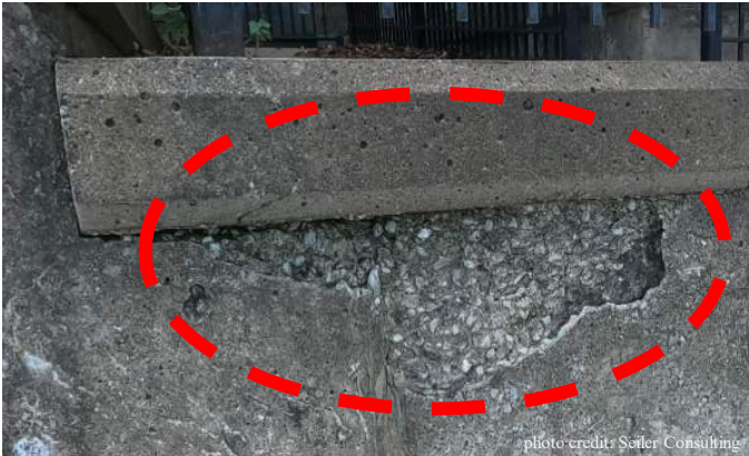
Spalling concrete sea wall
