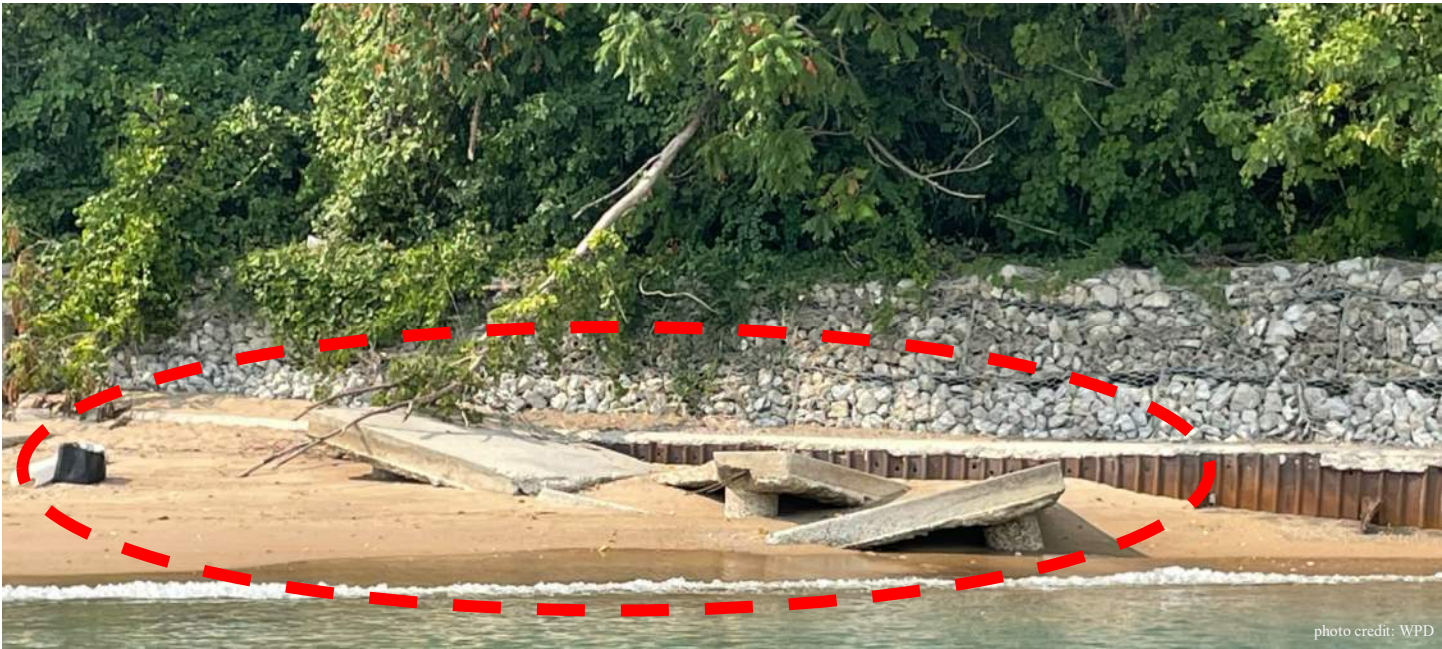
Damaged kayak storage rack foundations
