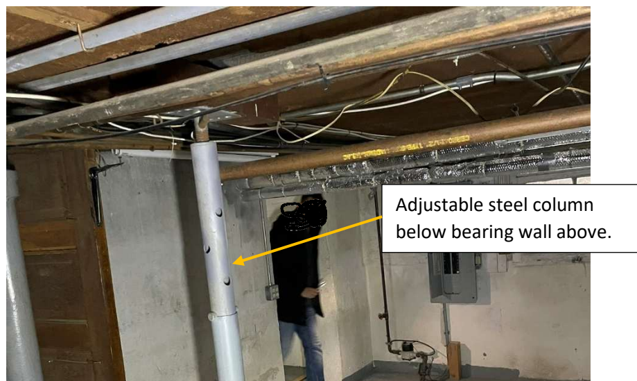
Picture 16: East Temporary Adjustable Column.
