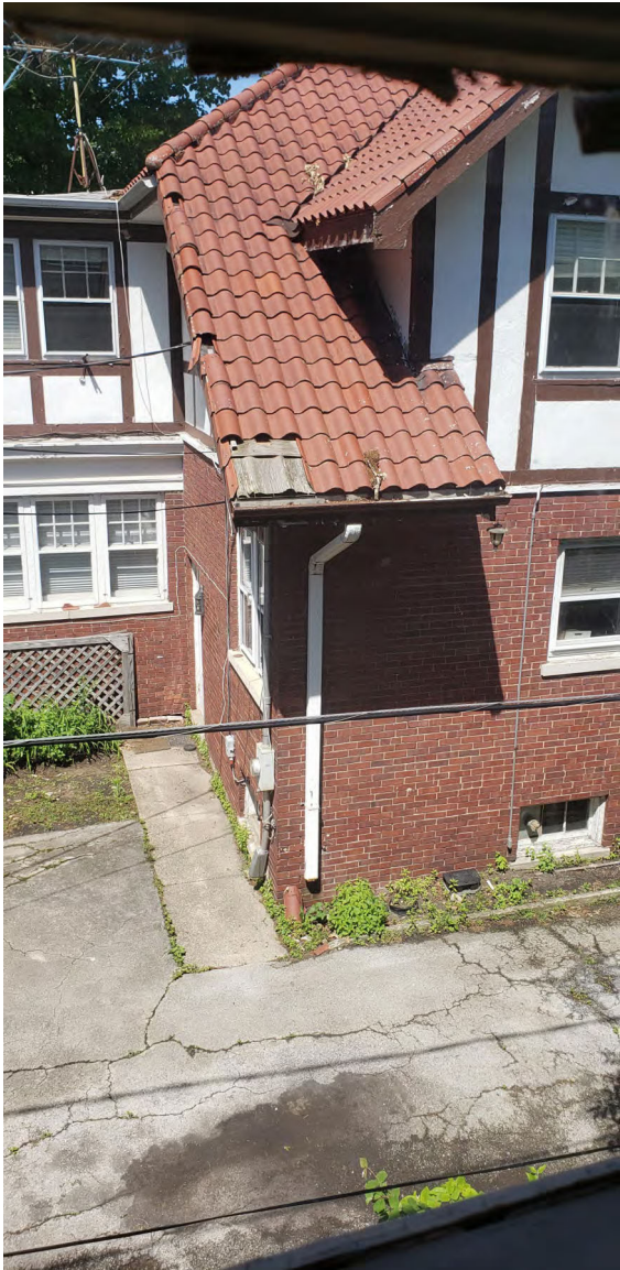
MISSING AND DAMAGED CLAY ROOF TILES
