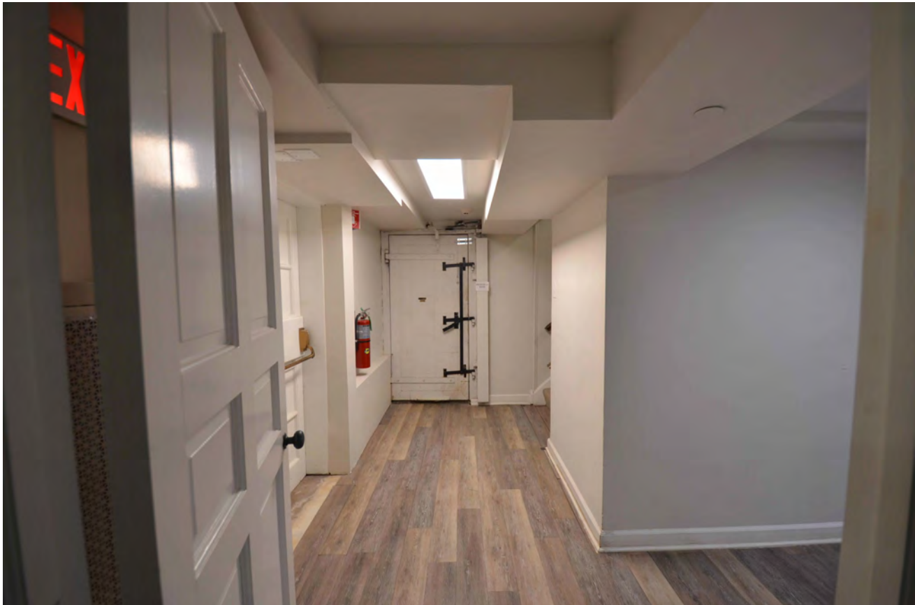
LIMITED HEADROOM IN EXISTING BASEMENT
