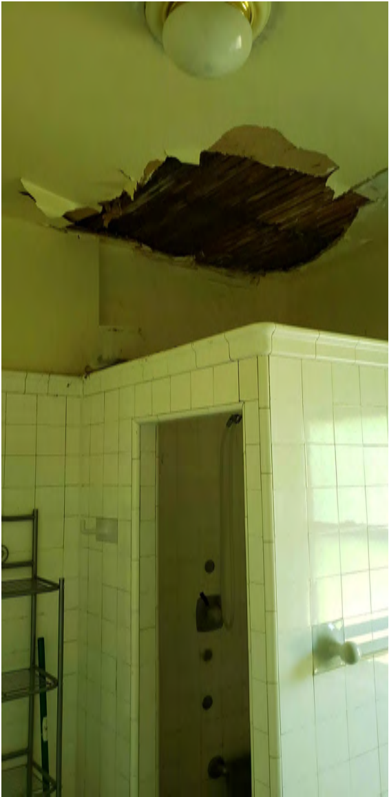
WATER DAMAGE AT FIRST FLOOR CEILING DUE TO DISREPAIR OF WATER LINES.
