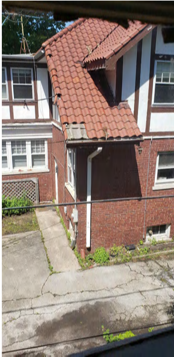
MISSING AND DAMAGED CLAY ROOF TILES
