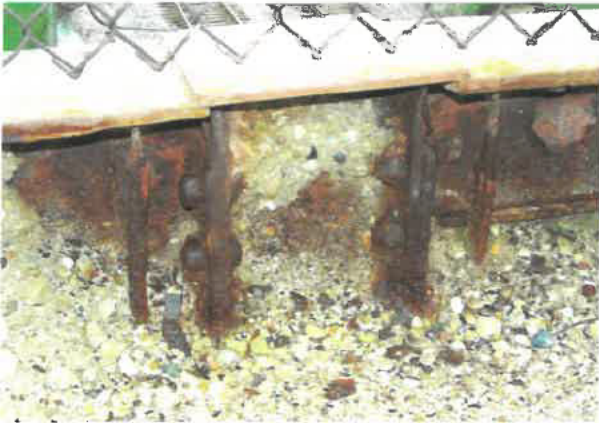
Figure 3 Typical corroded upper column bolted joint
