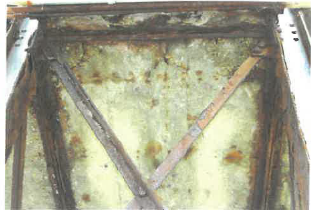
Figure 4 Typical corroded steel support framework
