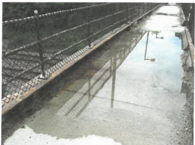
Figure 2 Pooling, missing concrete and exposed reinforcing
