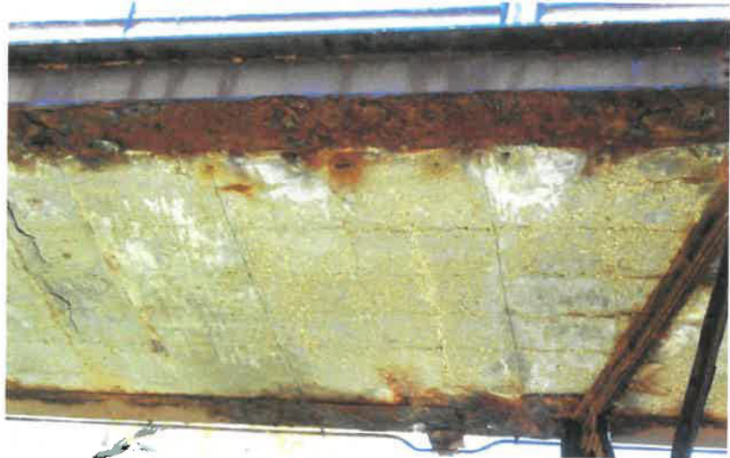
Figure 6 More details of corroded structure and failing concrete from below
