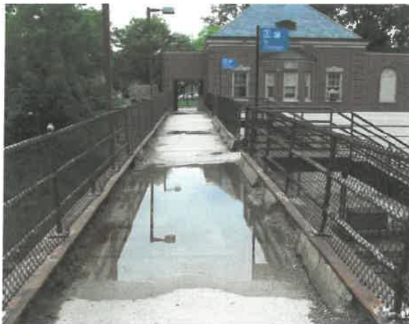
Figure 1 Hubbard Woods Bridge - sagged deck sections
