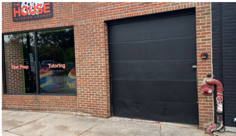
Figure 3 – The current front elevation of the future North Shore Barbershop, Mast Partners, LLC
