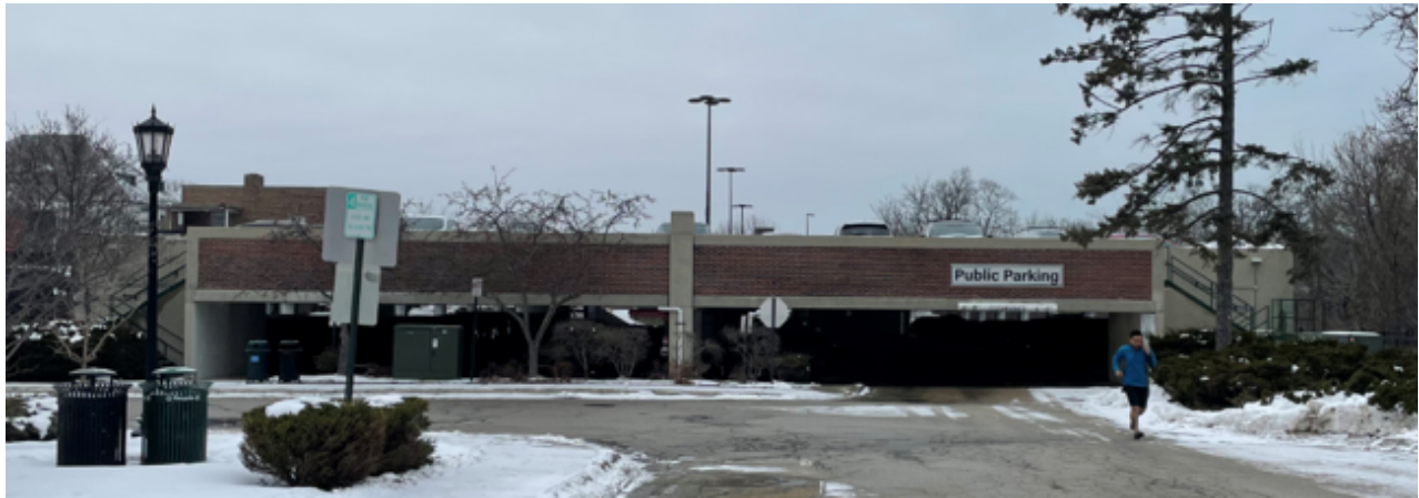
Figure 2 – Subject Property Public Parking Structure - South Entrance Elevation with existing wall sign
