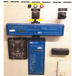
Critical information such as existing switchgear relay schemes will be confirmed onsite for inclusion into the new switchgear.
