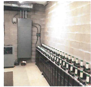
The existing switchgear battery backup system will be evaluated for the addition of the new switchgear control power loads.
