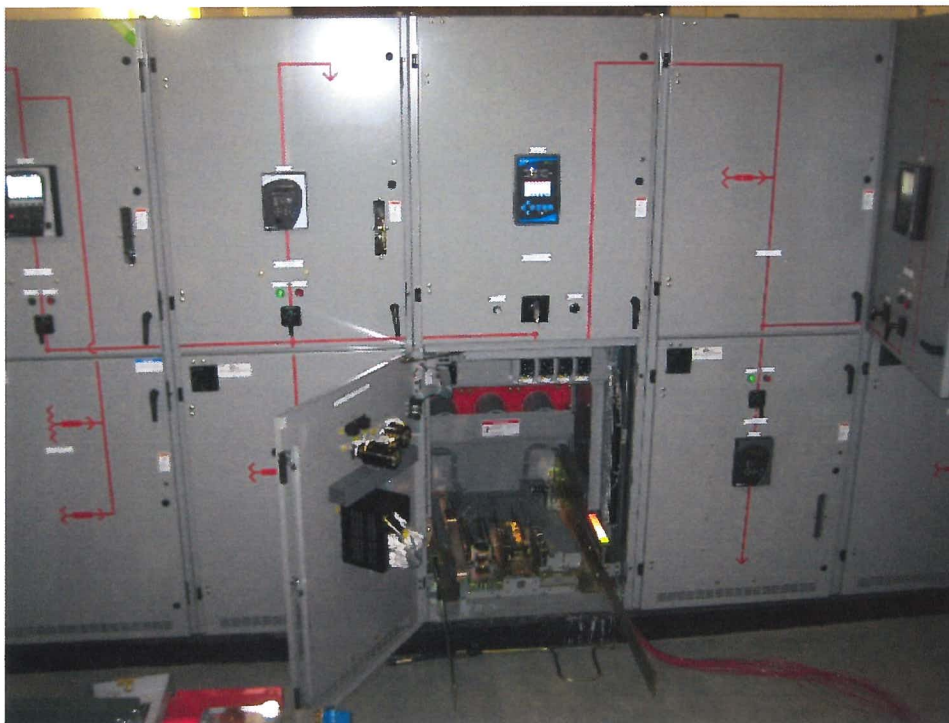
The new switchgear was tested onsite to confirm desired operation.
