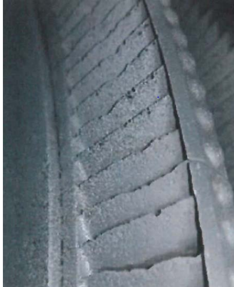
Photo of Blade Deterioration
