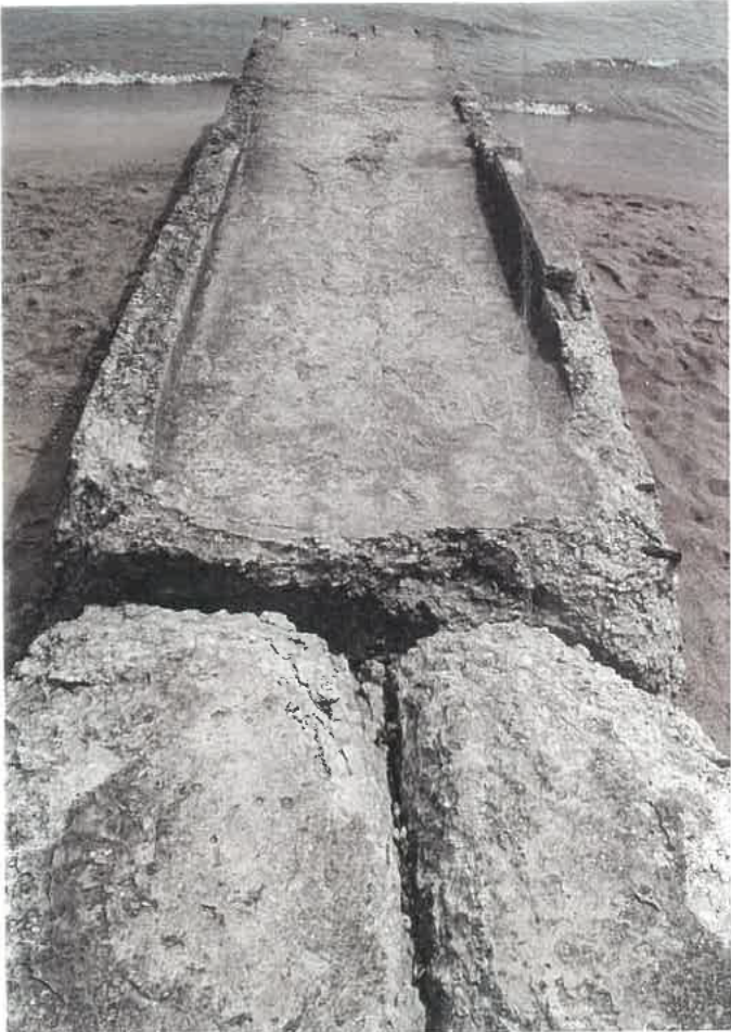
View of deteriorating pier.
