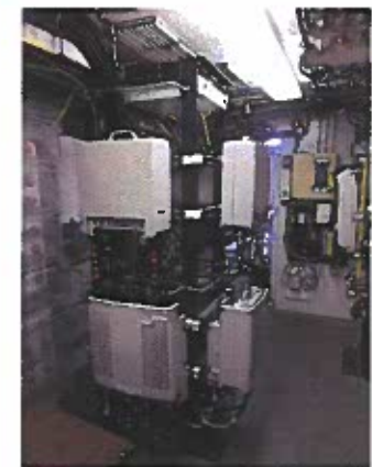
EXISTING LTE EQUIPMENT
