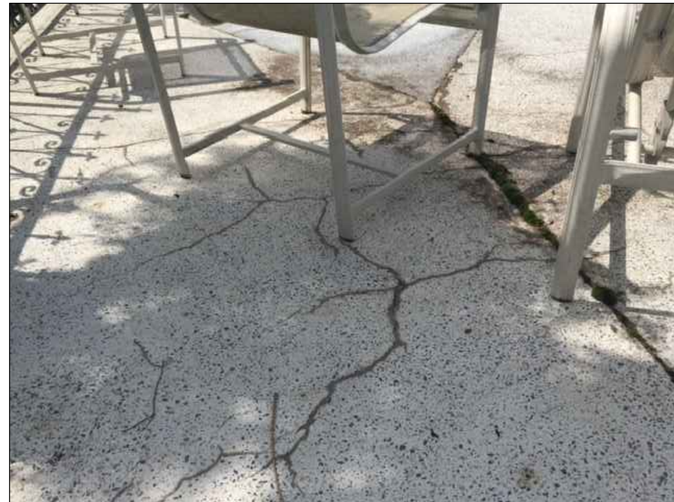
3 PHOTOS - EXISTING PAVERS CRACKED DUE TO MOISTURE Scale NO SCALE
