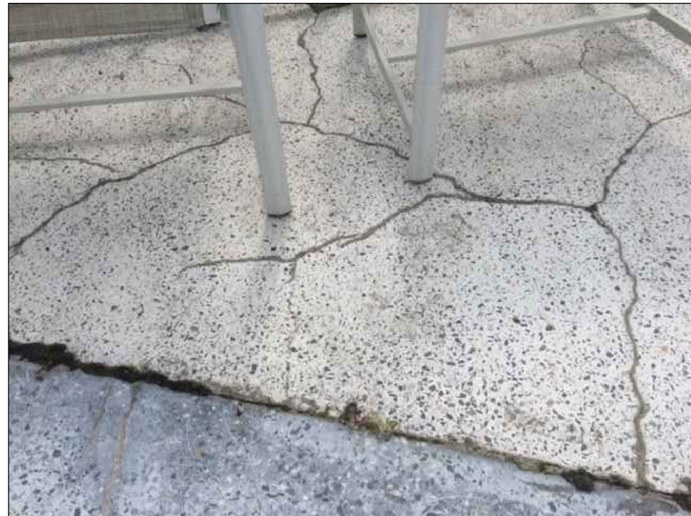
2 PHOTOS - EXISTING PADIO CRACKED DUE TO MOISTURE Scale NO SCALE
