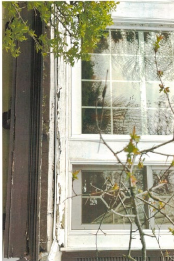
#11 WINDOWS & EXTERIOR DETERIORATED & NOT FIXABLE.
