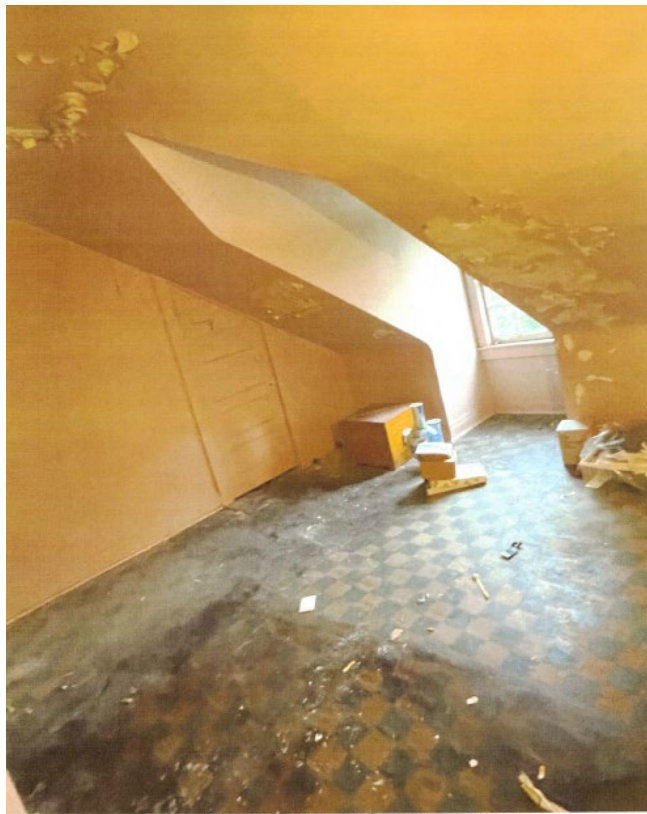
#9 DAMAGED CEILING IN THE ATTIC
