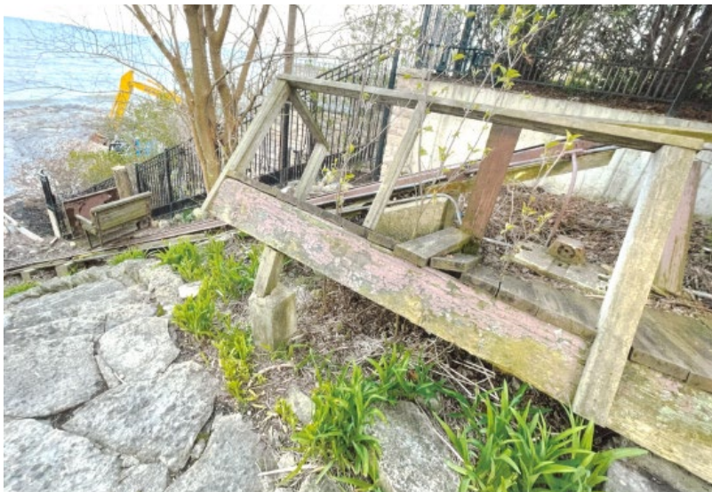
#13 BROKEN TRAM, ABANDONED AREA ON THE BLUFF
