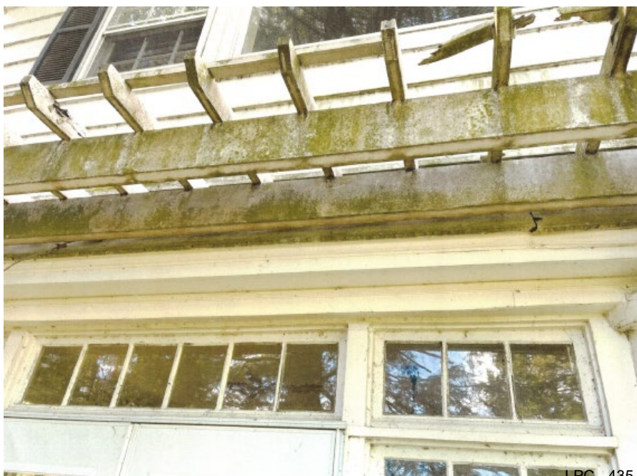
#14 DESTROYED, DAMAGED EXTERIOR
