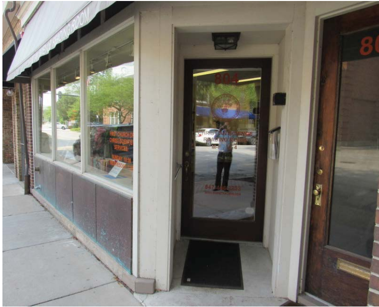
Figure 2 – Subject Property – Trim, door, and copper panels to be repainted, re-stained, and replaced.
