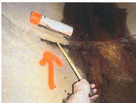
Figure 4.3: Marking pipe joint separation
