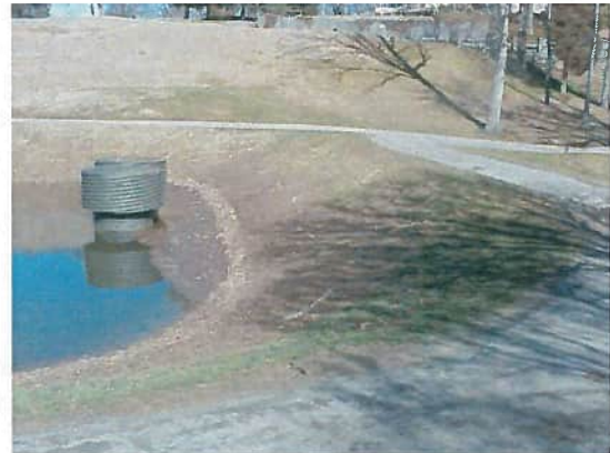
Figure 5.10: Bare soils on embankment and slopes
