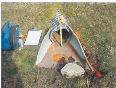
Figure 4.1: Marking outfall deficiencies.
