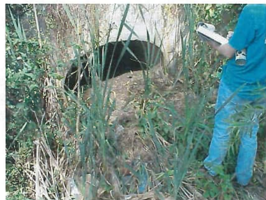
Figure 5.11: Excessive vegetation near an outfall
