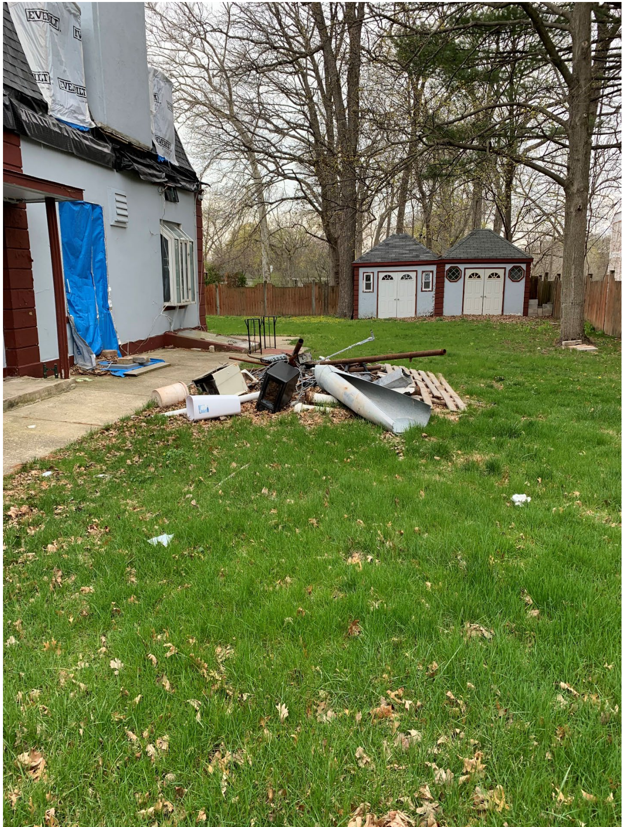
Figure 16 - site rubbish & debris
