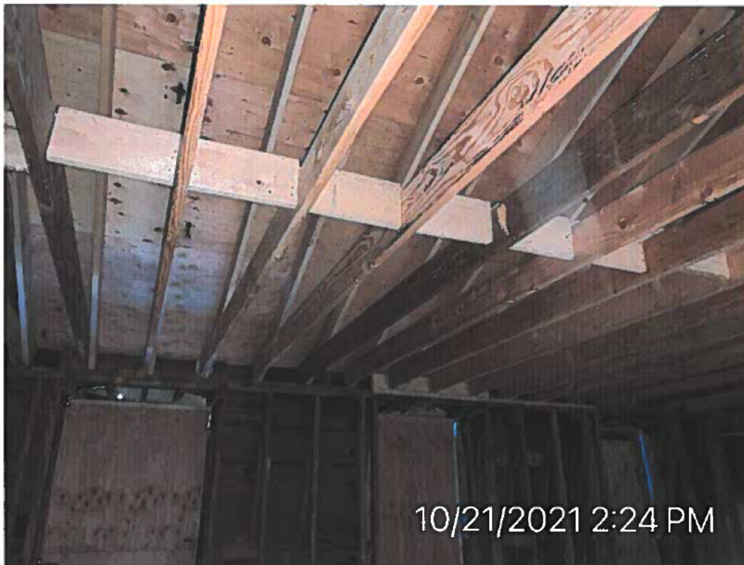
Unpermitted roof framing repairs from the interior of the home.
