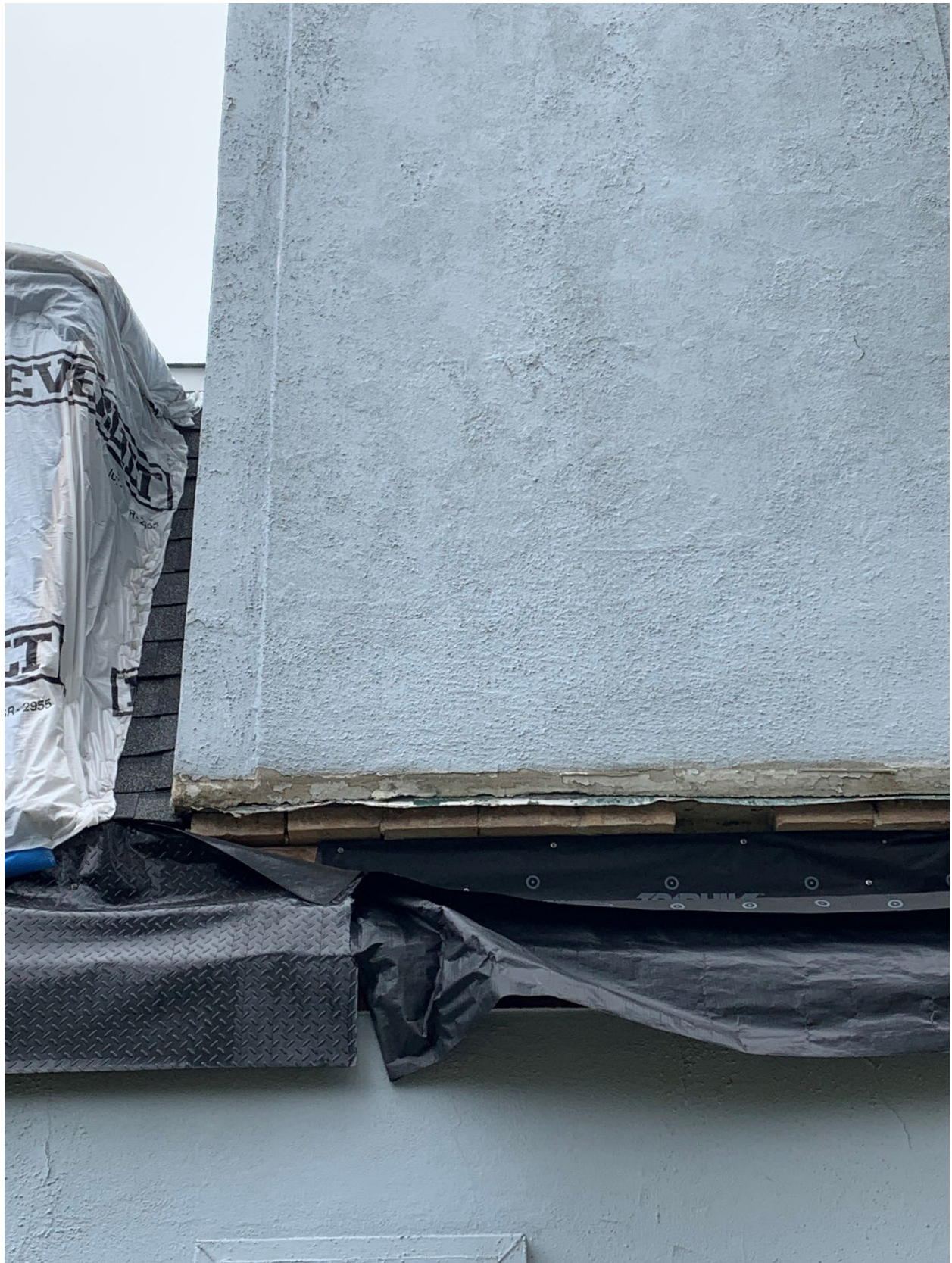
Figure 18 - exposed wood sheathing
