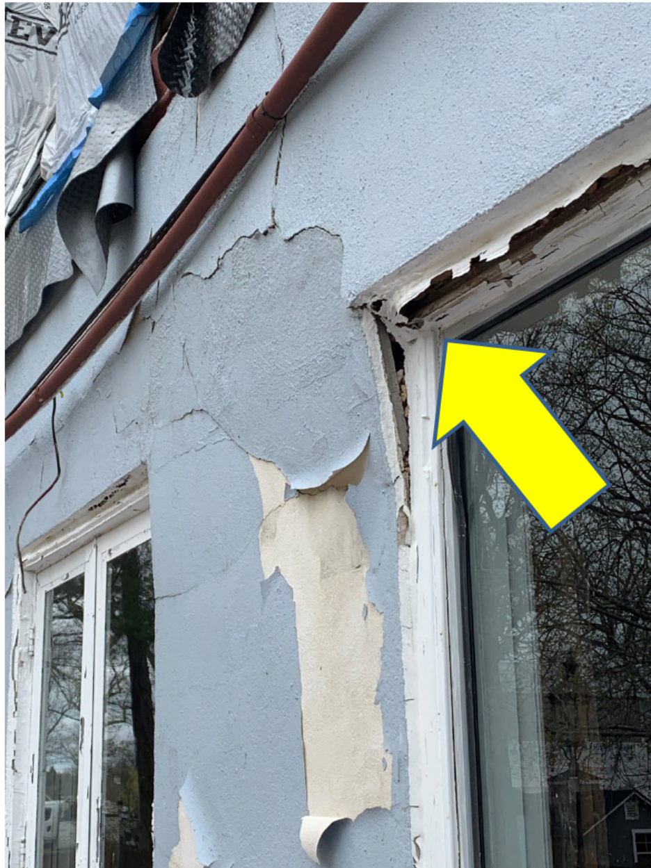
Figure 2 –stucco on west elevation pulled away from substrate
