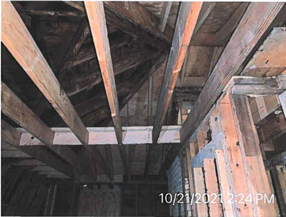
Unpermitted roof framing repairs from the interior of the home.
