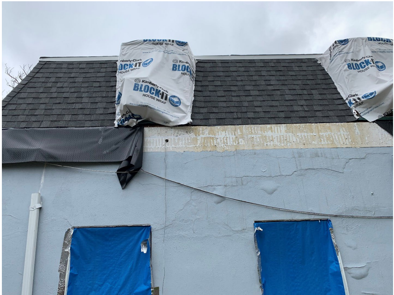
Figure 15 - missing/damaged temporary protection from water entry
