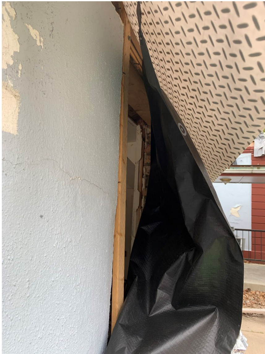
Figure 12 - unprotected garage opening
